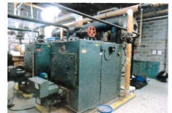
Existing Heating Hot Water Boilers
