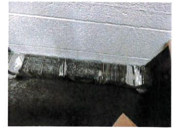
Inside Existing Hot Water Baseboard
