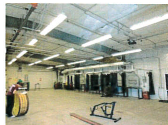
Existing Welding Area without Adequate Exhaust or Makeup Air
