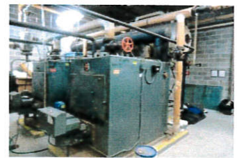
Existing Heating Hot Water Boilers
