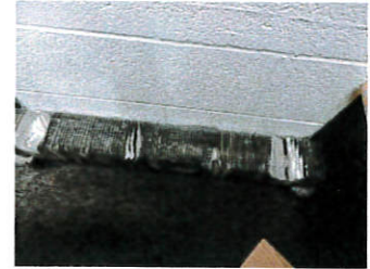
Inside Existing Hot Water Baseboard
