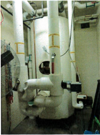
Existing Elementary School Indirect Domestic Hot Water Tank
