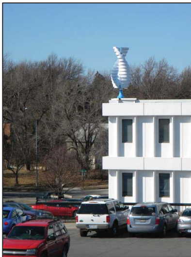
A Helix Wind Turbine on top of a Lincoln, Nebraska Office building.
