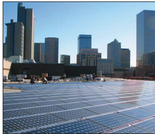
Solar panels on top of the Denver Convention Center.
