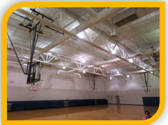
High Intensity Discharge Lighting
