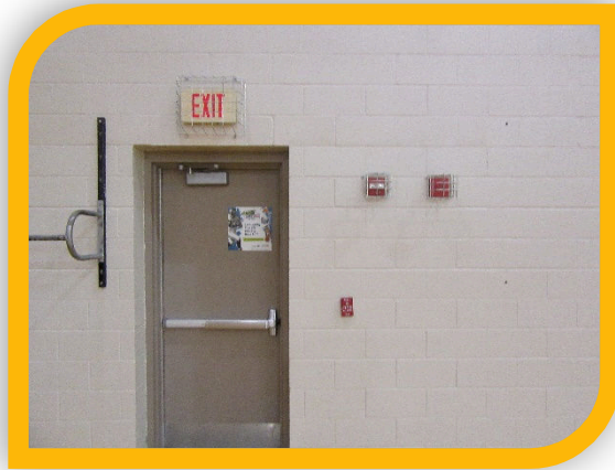
Bell, Strobe and Pull Station
