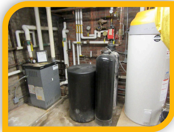
Domestic Hot Water Heater
