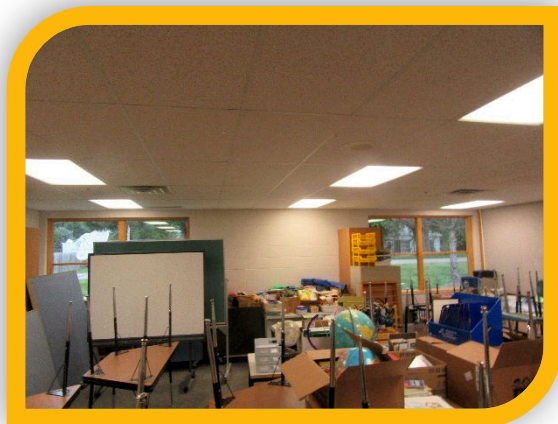
Fluorescent Lights and Suspended Ceiling
