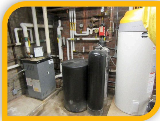
Hot Water Boiler
