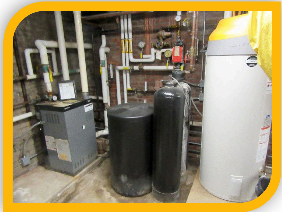
Water Softener System
