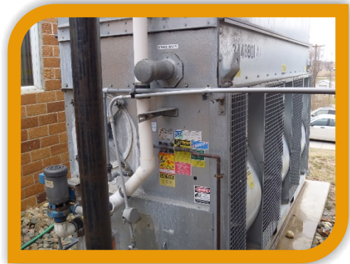
Heat Pump Fluid Cooler
