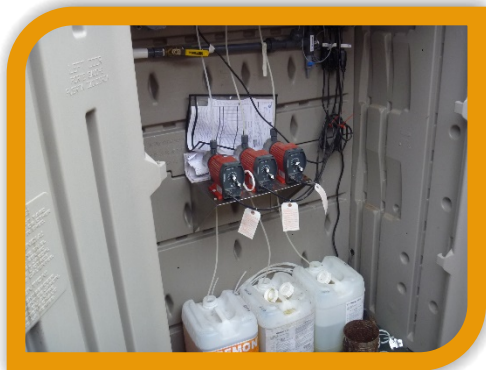
Fluid Cooler Chemical Feed System
