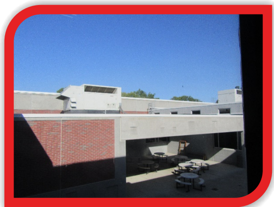
Roof Top Unit
