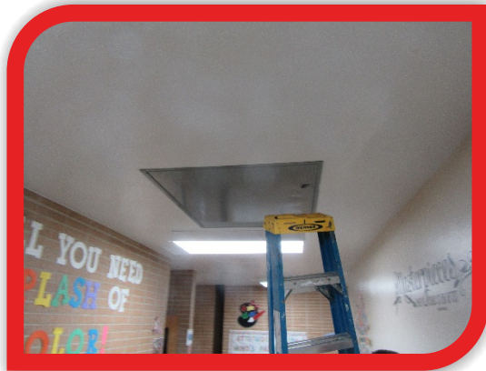
Elementary Mechanical Access
