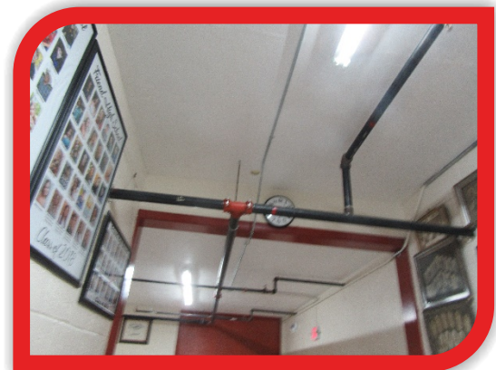
Fire Sprinkler System
