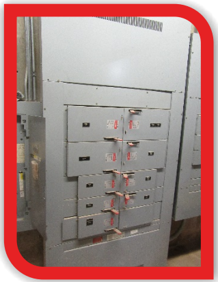
Main Distribution Panel
