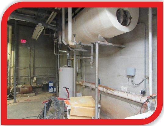
Hot Water Storage Tank
