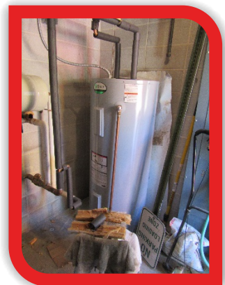
Elementary Water Heater
