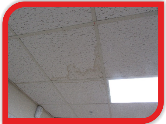
Elementary Water Stain
