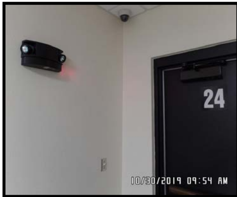
Door #24 emergency light non-operational High School
