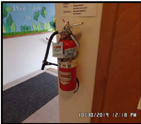
Out-dated inspection fire extinguisher Fisher School
