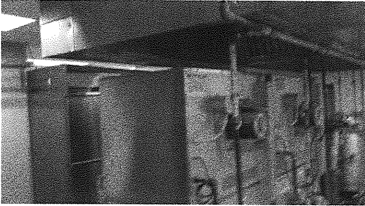
Kitchen equipment under hood.
