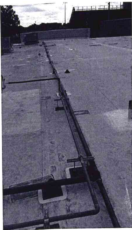
Unpainted gas piping and missing roof pad.
