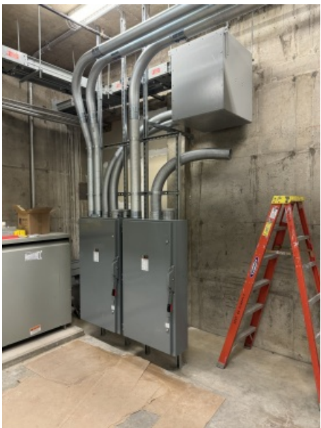
Part of getting the pool building ready for demo is the refeeding of the power serving the Geo Thermal Heat Pump Loop pumps and misc mechanical equipment. This picture is in one of the main Electrical Rooms near the main Gym. One temporary disconnect is for the Heat Pump Loop, and the other is for a new panel on 2nd floor by Tim's office.
