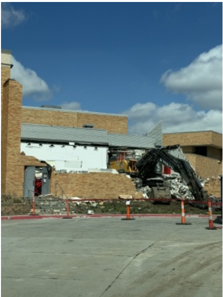
Peitzmeier Demolition used to back hoes to take down the roof structure of the Blue Gym. Picture taken on 4/3. They are hauling out the separated concrete and steel daily as the take the building down.
