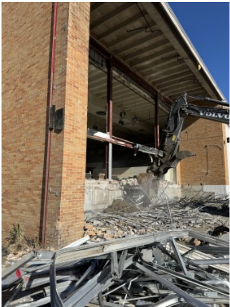
Also getting started into the pool area. Weitz's goal is to start the Building demo of the pool area the week of 4/22.
