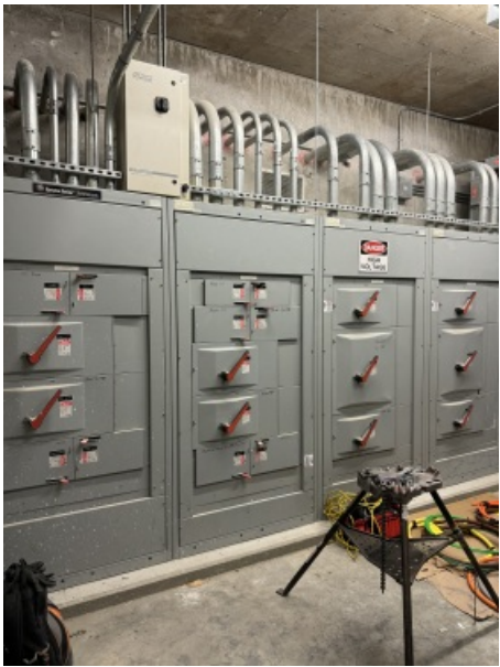
The existing gear serving the old pool building.
