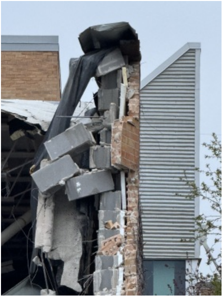
Typical wall section of the old Blue Gym had foam insulation in the cavity between the CMU wall and the Brick veneer.
