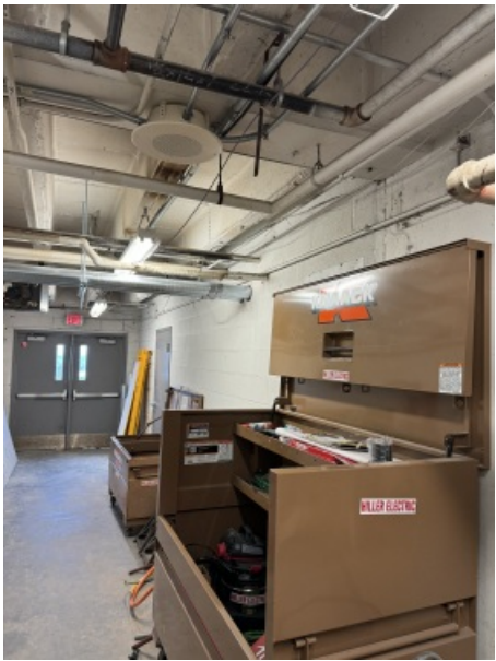
Another picture documenting the conduit path in the basement.
