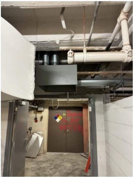
Junction Box for the feeds to the Geo Thermal Pump Equipment.
