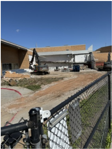
Getting ready to take out the stairs between Blue Gym and the pool. Early week of 4/8.
