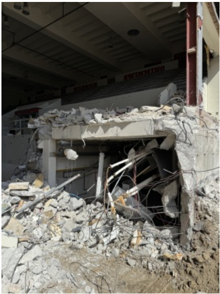
Looking North into the basement Mechanical Room of the Pool area.
