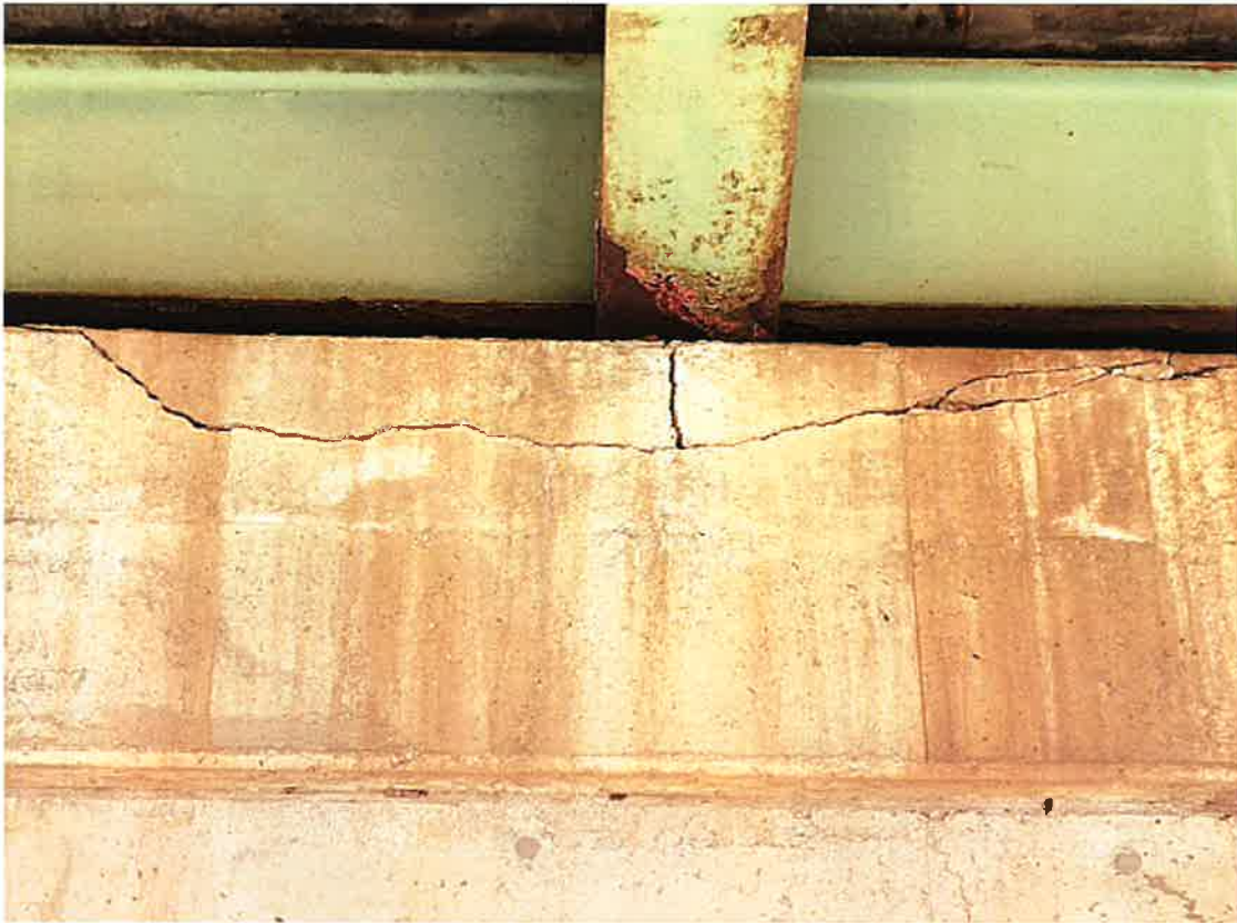
Cracking on the far side of Pier #6 cap under Girder #4.
