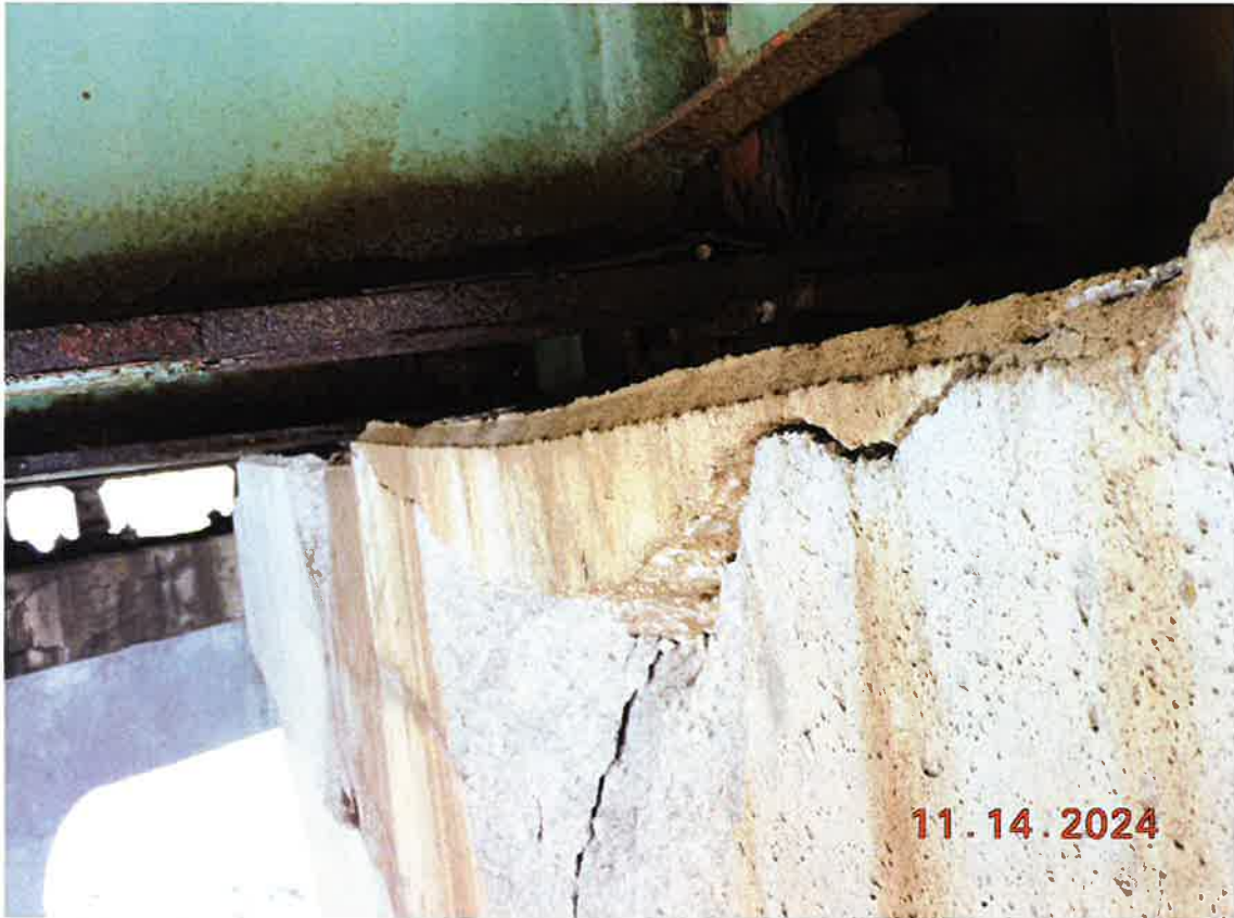
N face of Pier #6 at Girder #5. This is in the center of the inside traffic lane. Note the difference in staining between the upper portion of the spall and the lower portion. Also note the movement of the upper spall, translating N.
