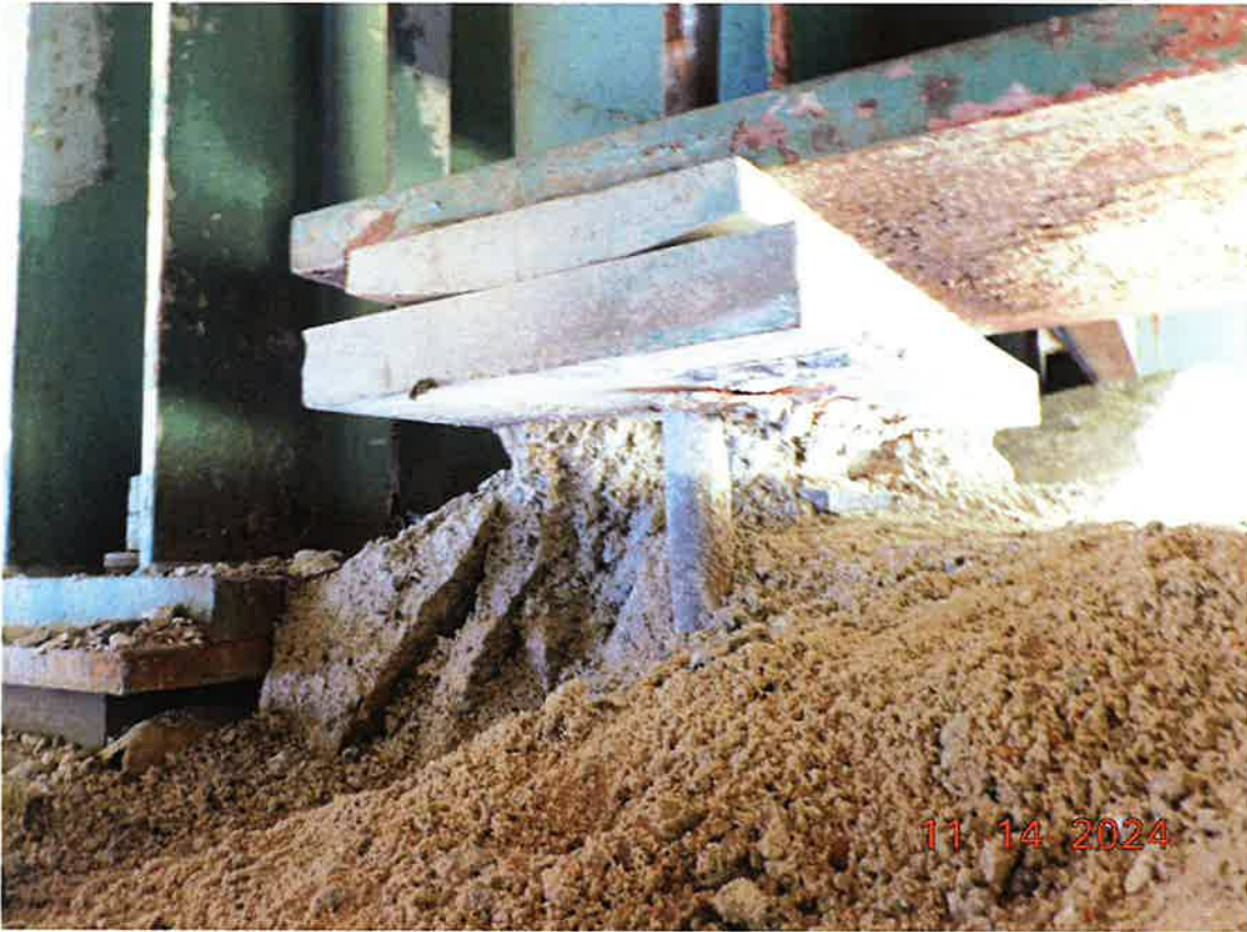
Pier #6, Girder #7 bearing area after unsound concrete is cleared away. No sound bearing material remains.
