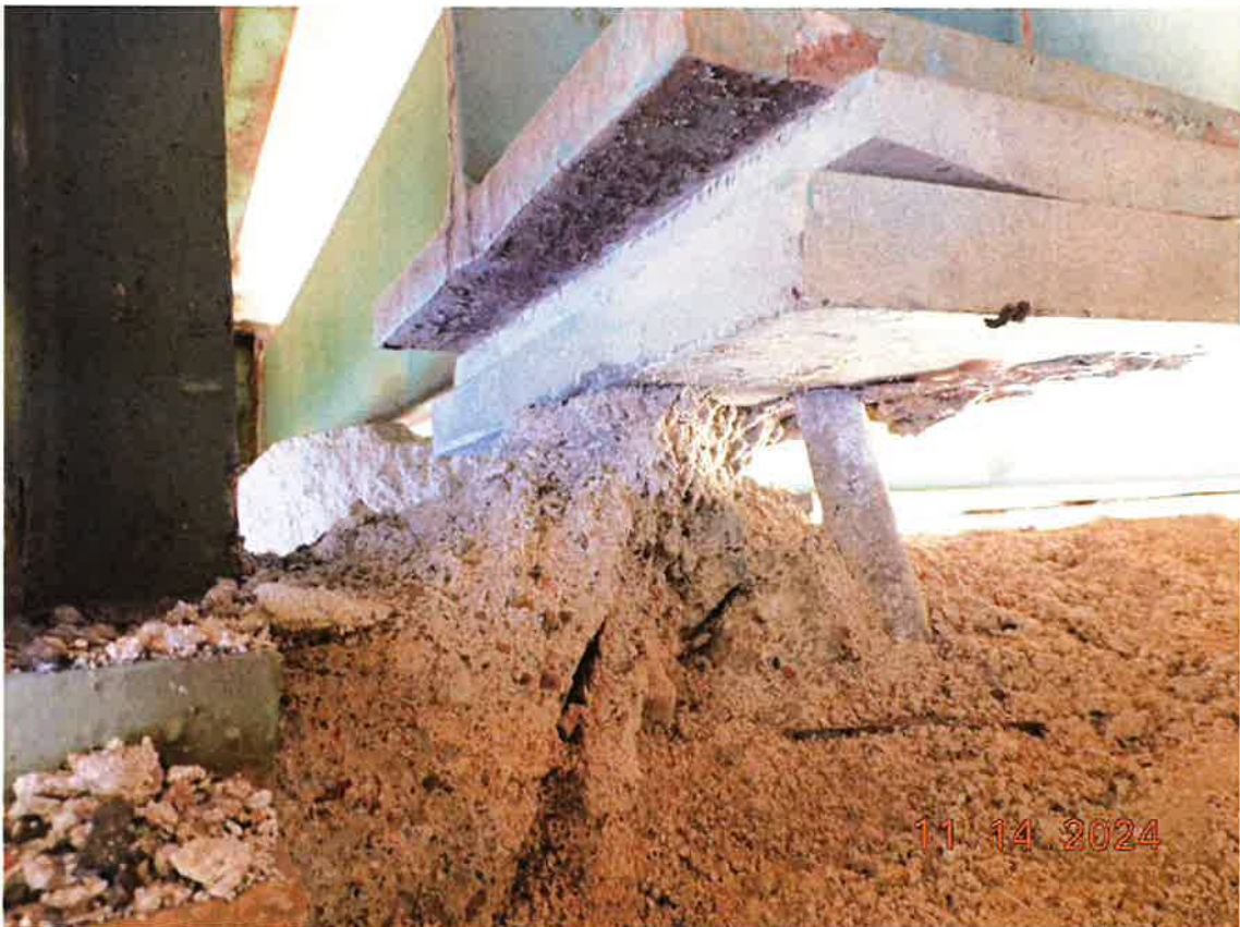
Pier #6, Girder #7 bearing area looking NW after unsound concrete is cleared away. No sound bearing material remains.
