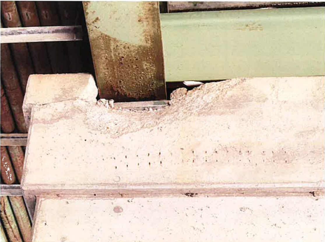
Spalling on the far side of Pier #6 cap under Girder #7.
