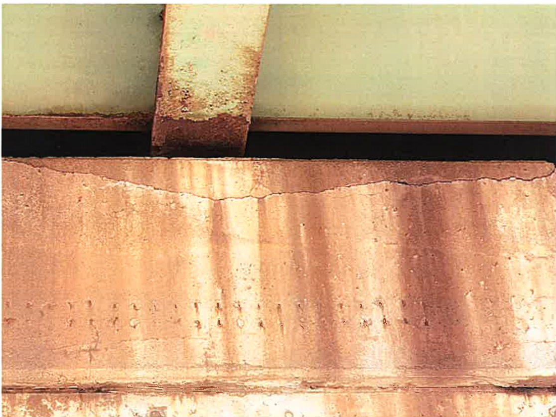
Cracking on the far side of Pier #6 cap under Girder #3.
