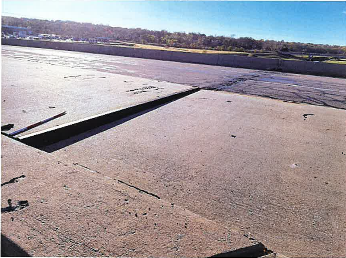
The SE corner of Span #7 has dropped above Pier #6.
