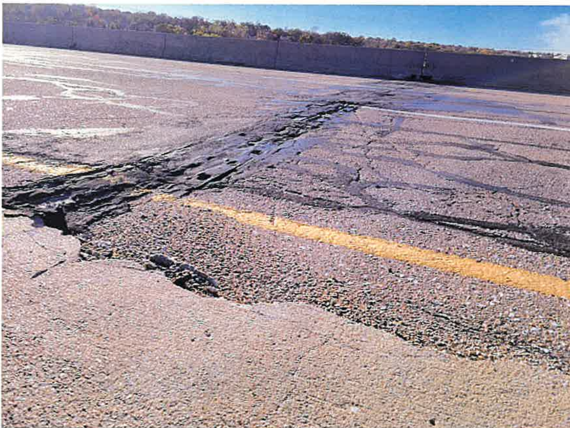
The east lane has dropped 2.5" at the curb and 0" at the west edge of the lane.
