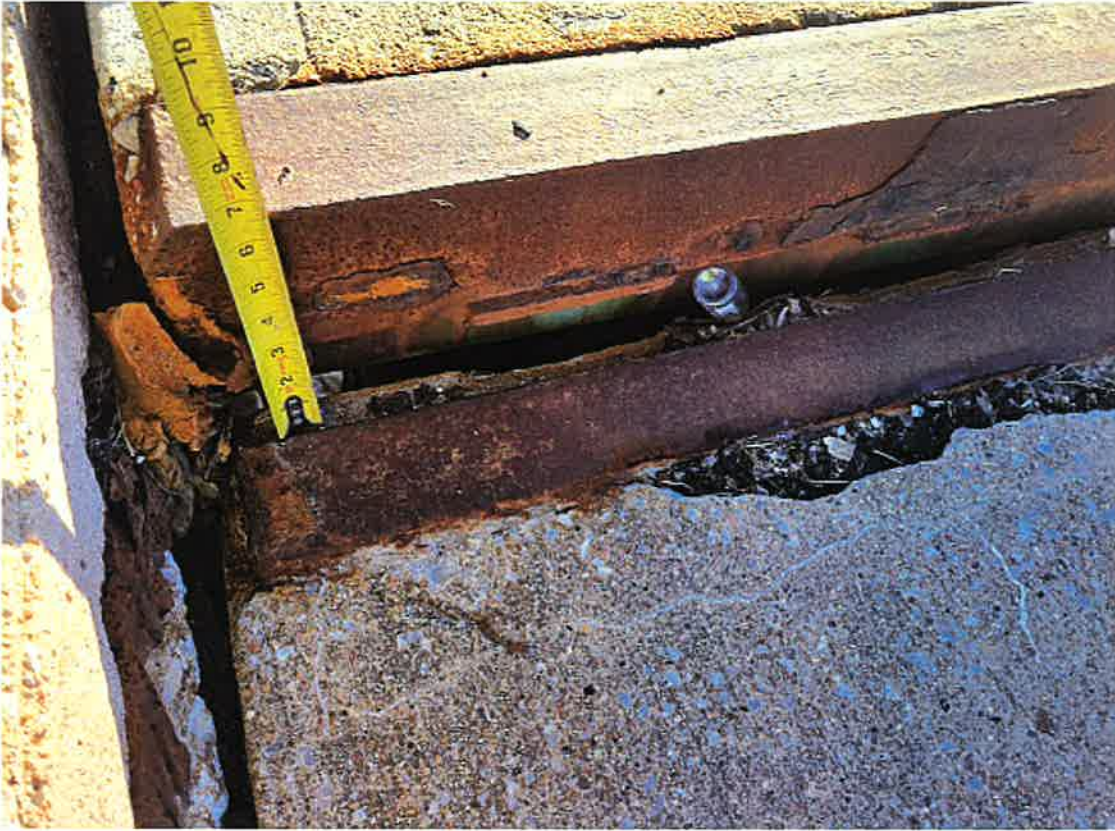
Deck has dropped 7" at the east edge.
