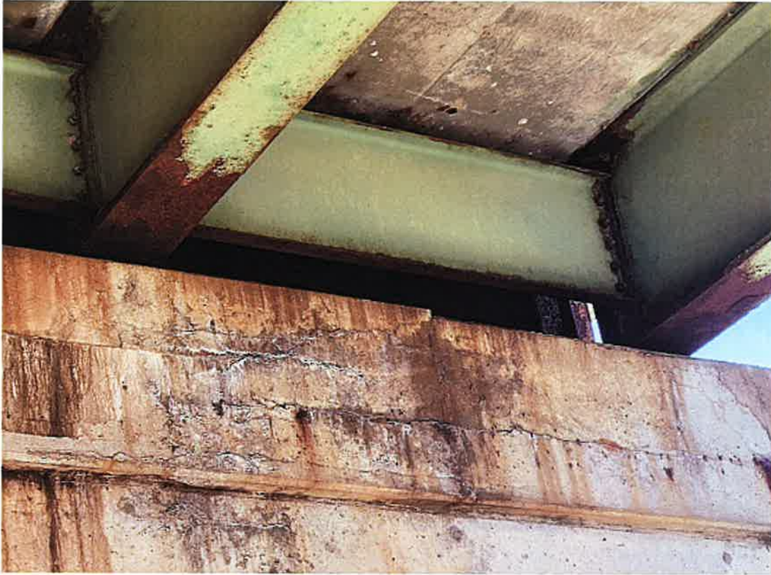
Cracking on the far side of Pier #6 cap under Girder # 2 and #1.
