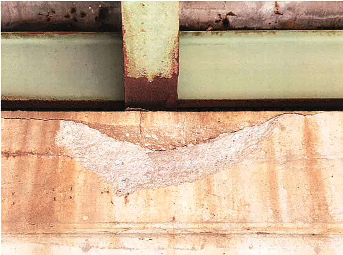
Spalling on the far side of Pier #6 cap under Girder #5.
