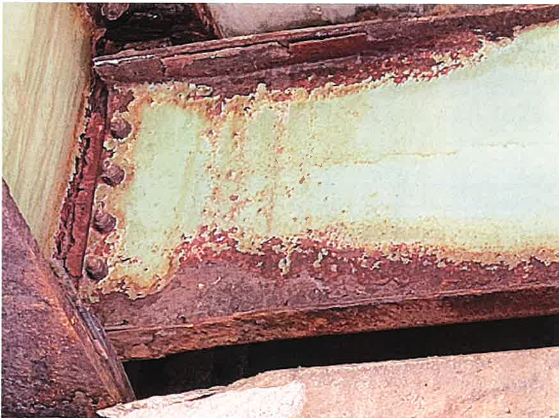
Diaphragm between Girder #5 and #6 appears to be bending near Girder #6 above Pier
