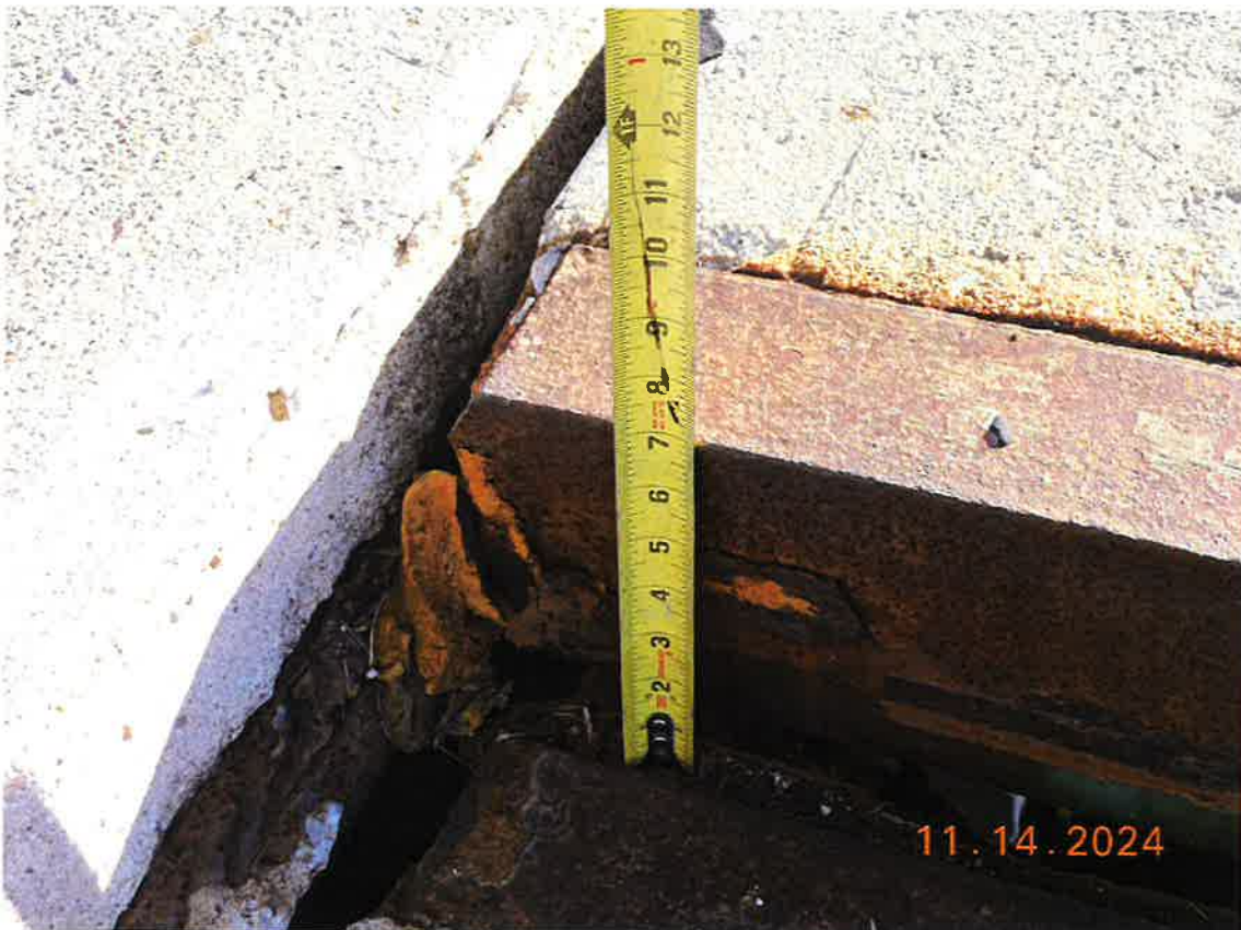
Differential settlement at the E end of the median joint at Pier #6.
