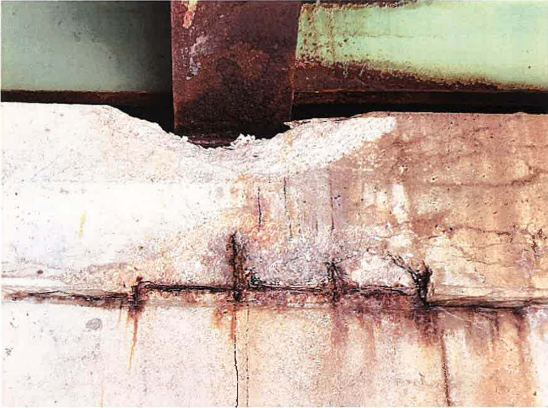
Spalling on the far side of Pier #6 cap under Girder #6.
