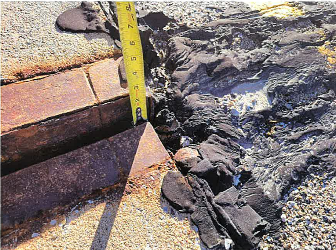
Deck has dropped 2.5" at the east curb.
