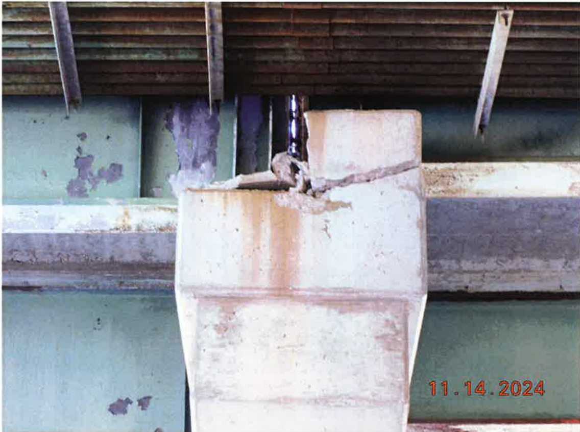
End view of E end of Pier #6 cap. The higher step on the right side of the cap supports the simple span girder in Span #7. The step is broken and there is no reinforcement tying the step to the pier cap.
