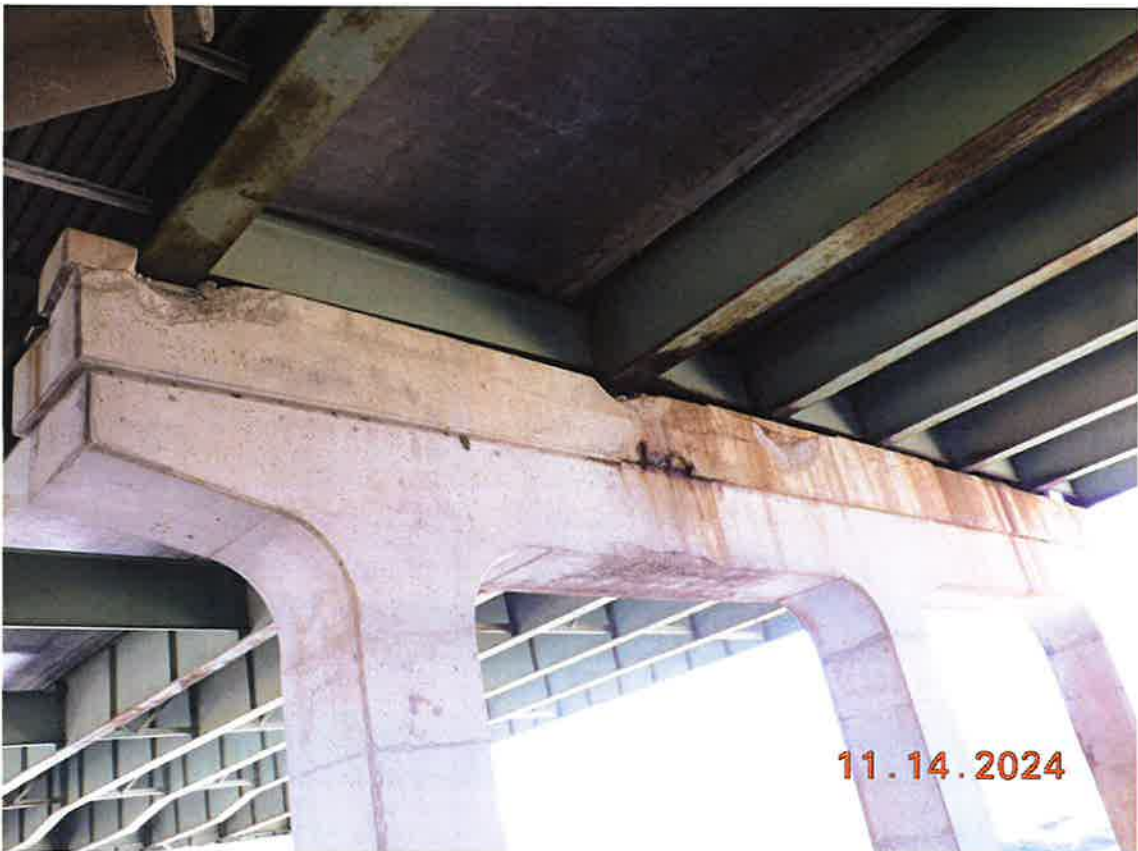
N face of Pier #6 looking SW. Girder #7 is in the foreground, Girder #1 is in the background.
