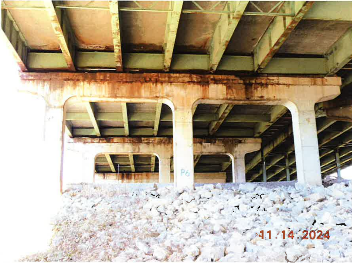
S face of Pier # 6. Girder #1 is left, girder #7 is right. Note staining from leaking joint at this pier.
