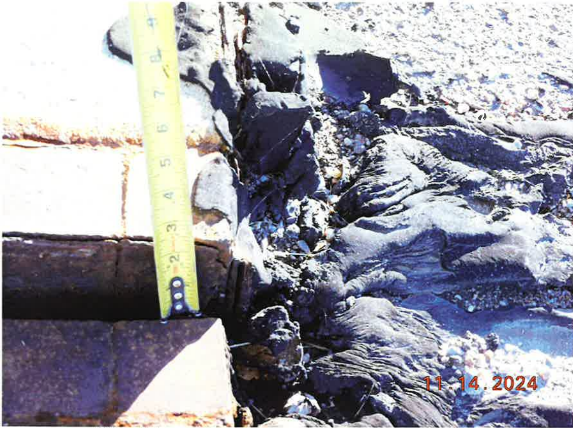
Differential settlement at the W end of the median joint at Pier #6
