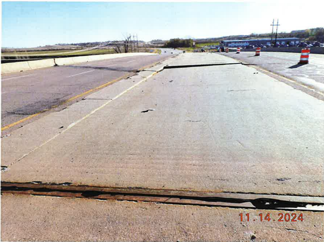
Median view looking S. Note differential settlement at the joint in the background, this is the joint at Pier #6.
