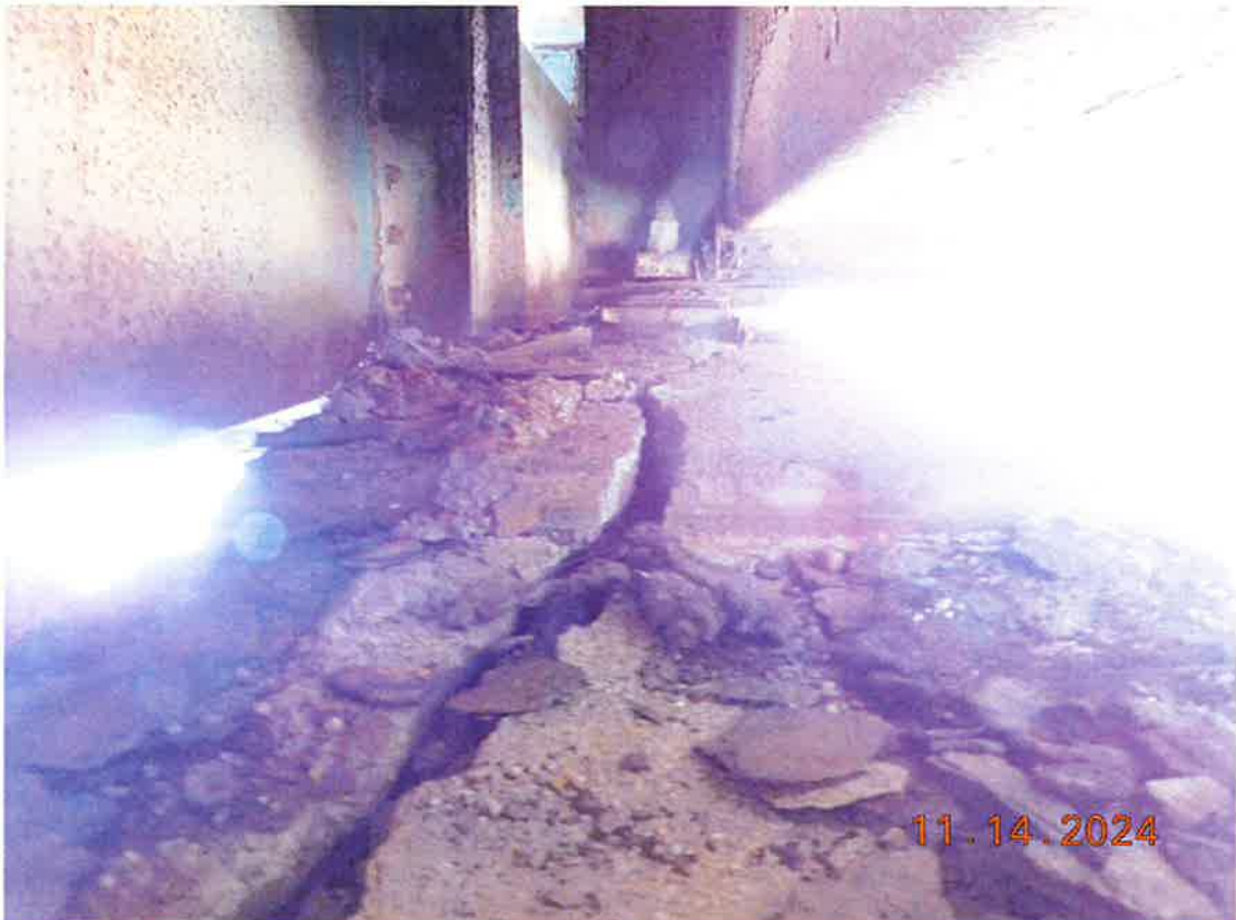
Pier #6, view of cap from the top looking W. Note large longitudinal crack in the unreinforced step for the simple span girders.
