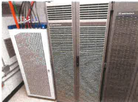
EQUIPMENT INSIDE SHELTER SCALE: NTS
