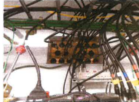
COAX PORT INSIDE SHELTER SCALE: NTS
