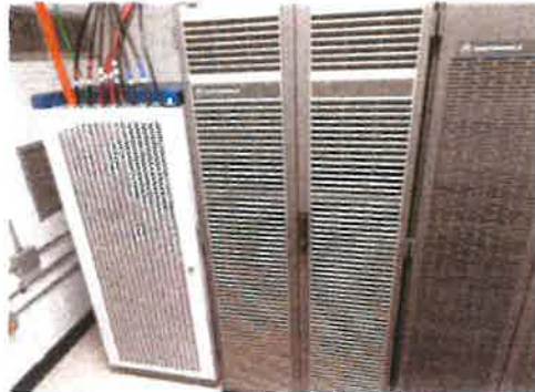
EQUIPMENT INSIDE SHELTER SCALE: NTS
