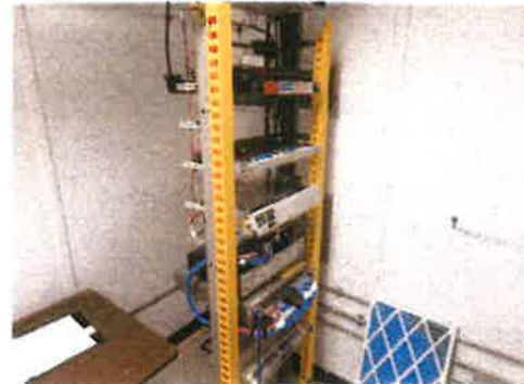
EQUIPMENT INSIDE SHELTER SCALE: NTS
