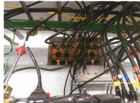
COAX PORT INSIDE SHELTER SCALE: NTS
