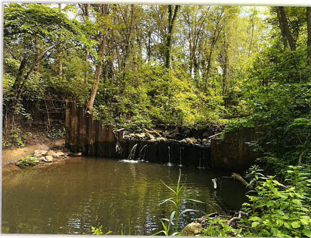
Photograph 1: Existing failing drop structure downstream of S 25 th Street
