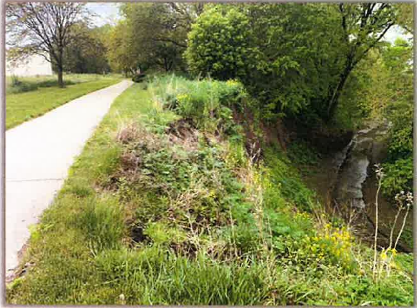
Photograph 2. Channel Widening and Meandering Banks Encroach on Nearby Trail
