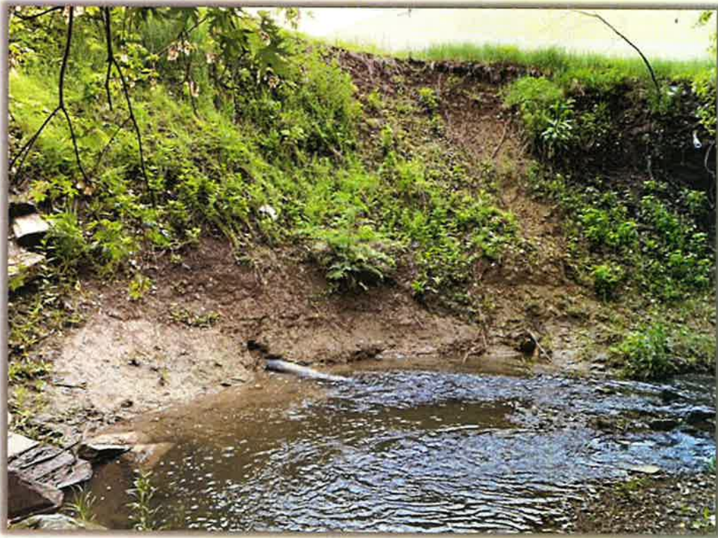
Photograph 3. Exposed Sanitary Sewer Line
