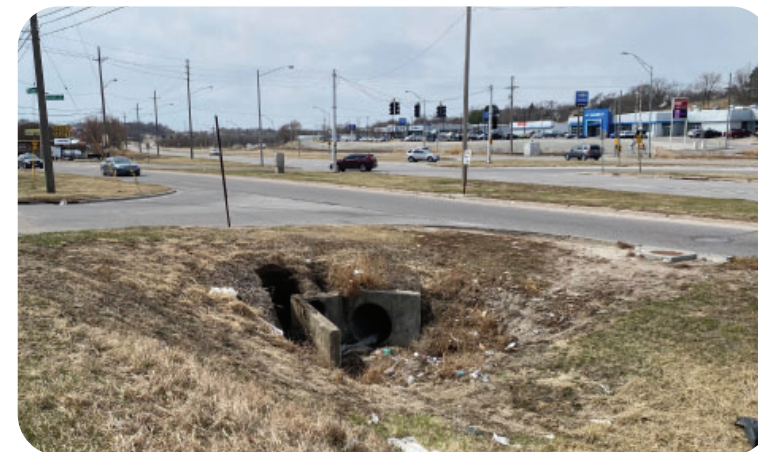
Deteriorating sewer near the Galvin & Fort Crook Roads intersection
