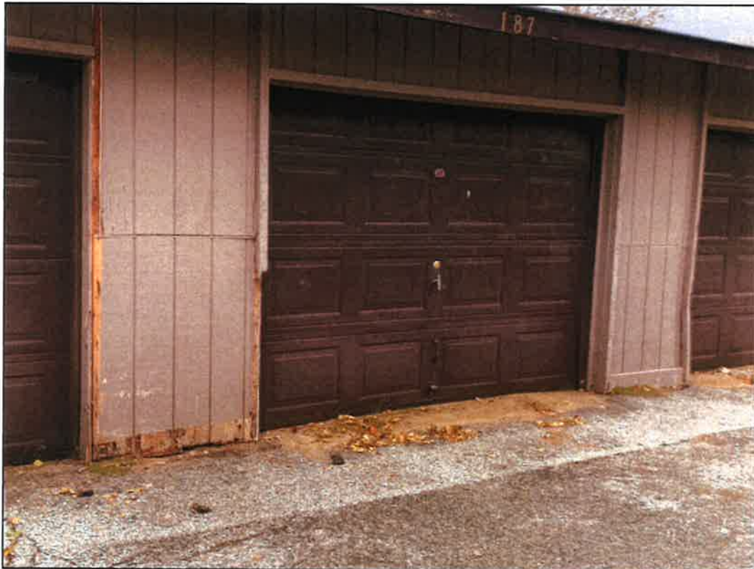
Poor garage maintenance
