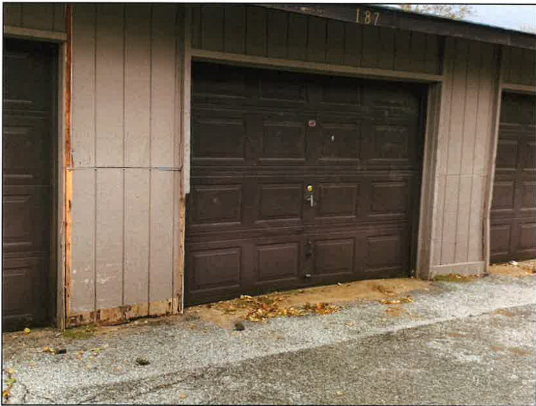
Poor garage maintenance
