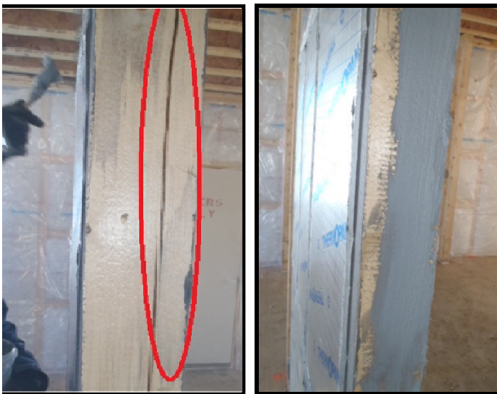
Wood is an imperfect material: a full-length check in this framing material leaked & was sealed
