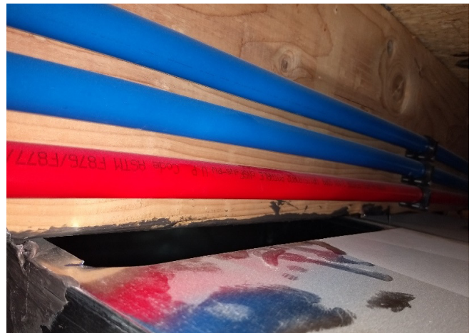
This 2-inch overcut was not visible from below & was difficult to seal
