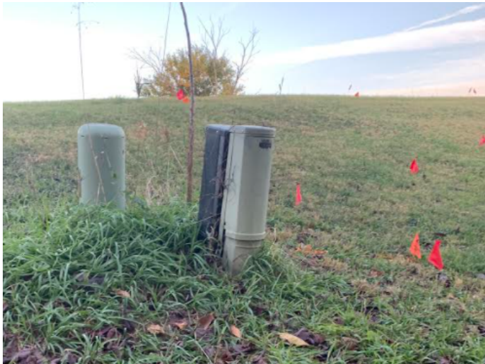
Image 4: This picture shows the junction box on the north side of Lot 13 and south side of Lot 12
