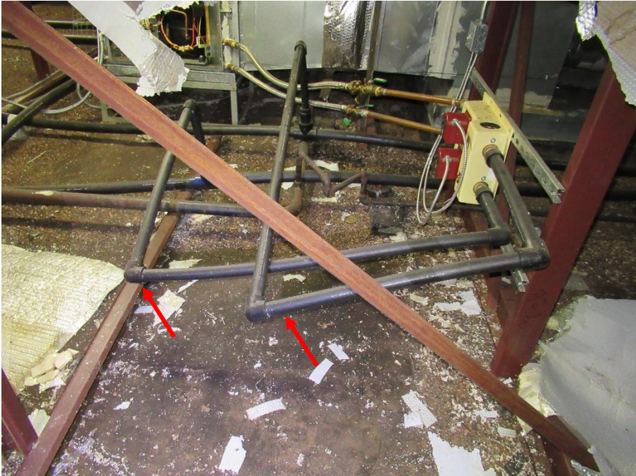
Photo 8 – Insufficiently supported piping
