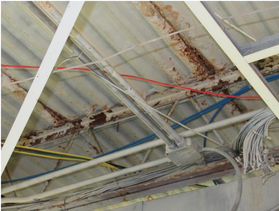
Photo 15 – Corrosion at metal roof deck and steel joists
