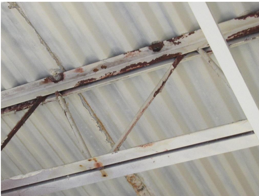
Photo 14 - Corrosion at steel joists
