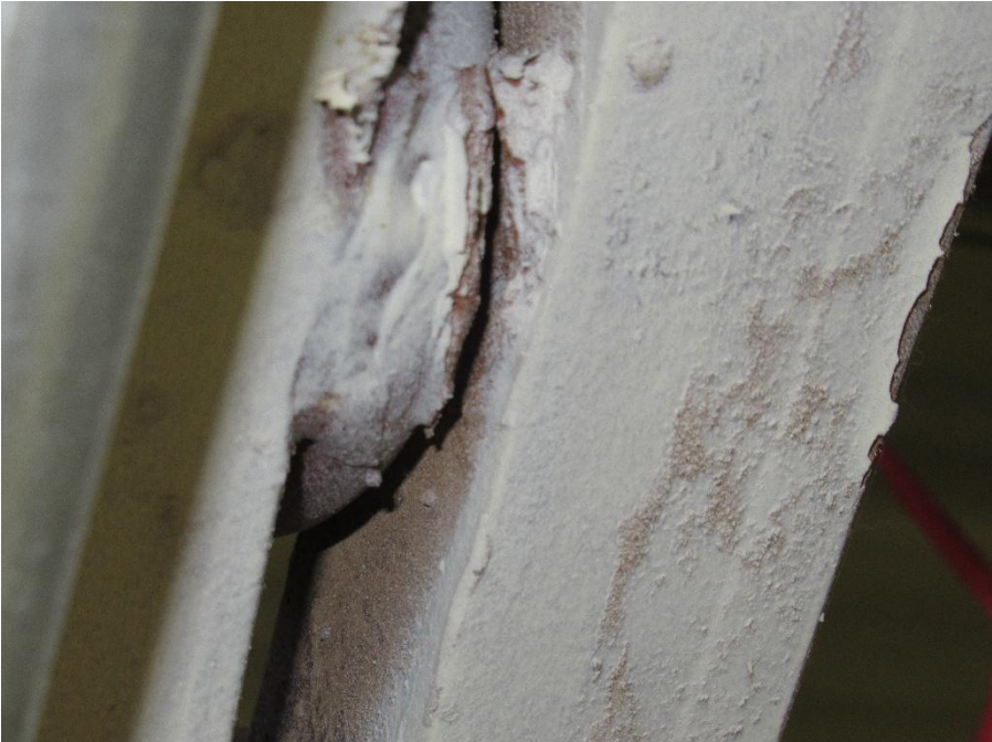
Photo 12 - Close up of broken weld in Photo 11
