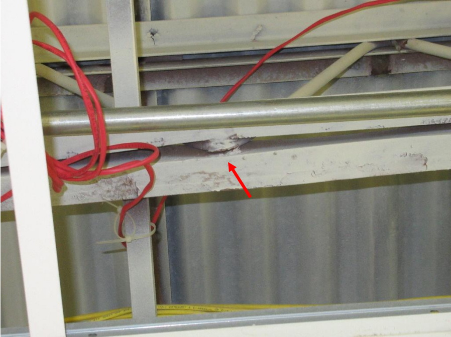
Photo 11 - Broken weld at steel joist web to bottom chord connection
