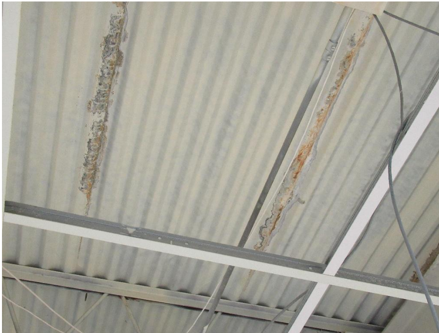
Photo 13 - Moisture migration through metal roof deck side laps
