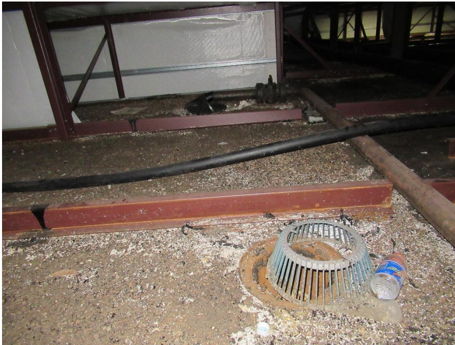
Photo 9 - Staining and discoloration of original roofing
