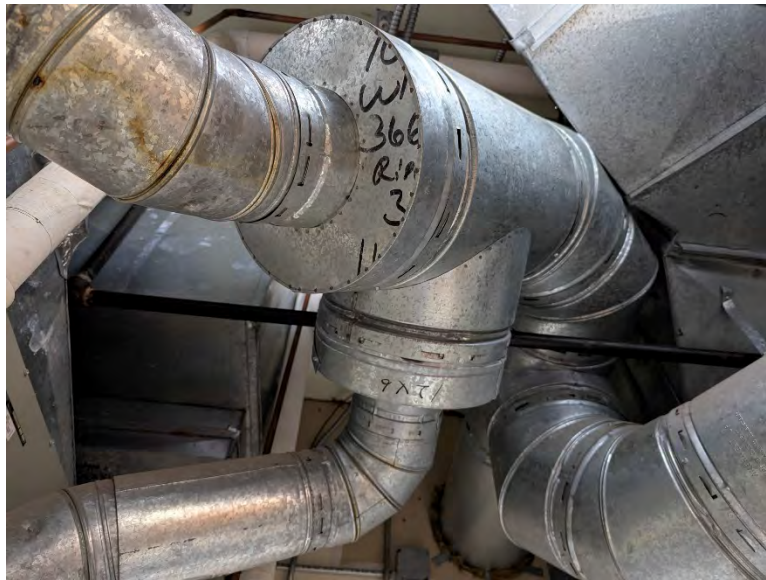
Figure 8. Various ducts tied to vertical air handlers
