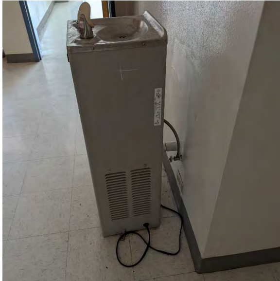
Figure 5. Typical drinking fountain
