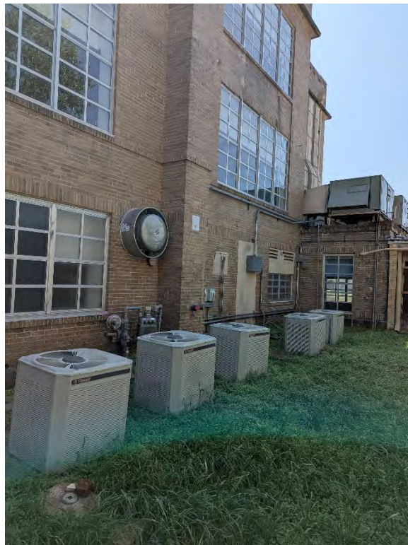
Figure 10. First floor outdoor units in mechanical yard
