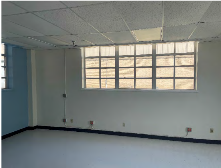
Figure 83. Typical wall showing orange isolated ground receptacles and surface mounted raceway
