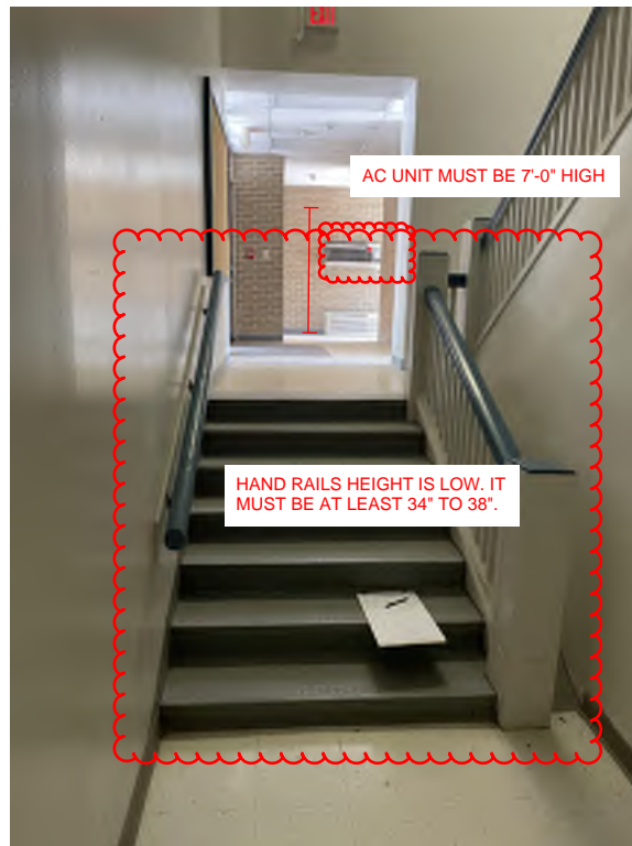
Figure 9: Stair handrails & AC unit not ADA complaint
