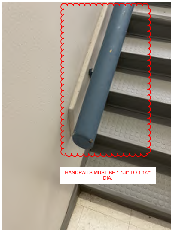
Figure 8: Stair handrails in First Floor Basement
