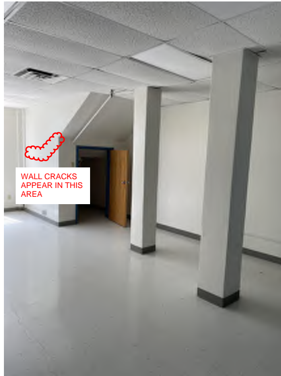
Figure 13: First Floor Basement Cracked Walls
