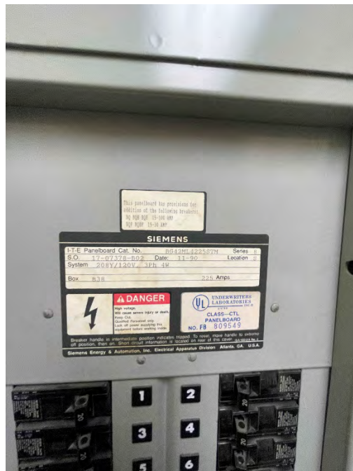
Figure 17. Panelboard nameplate showing a date of 1990
