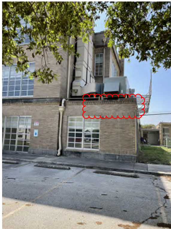
Figure 4: Repoint minor cracking of brick
