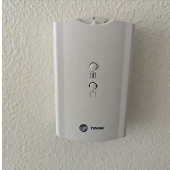
Figure 9. Second floor standalone control thermostat
