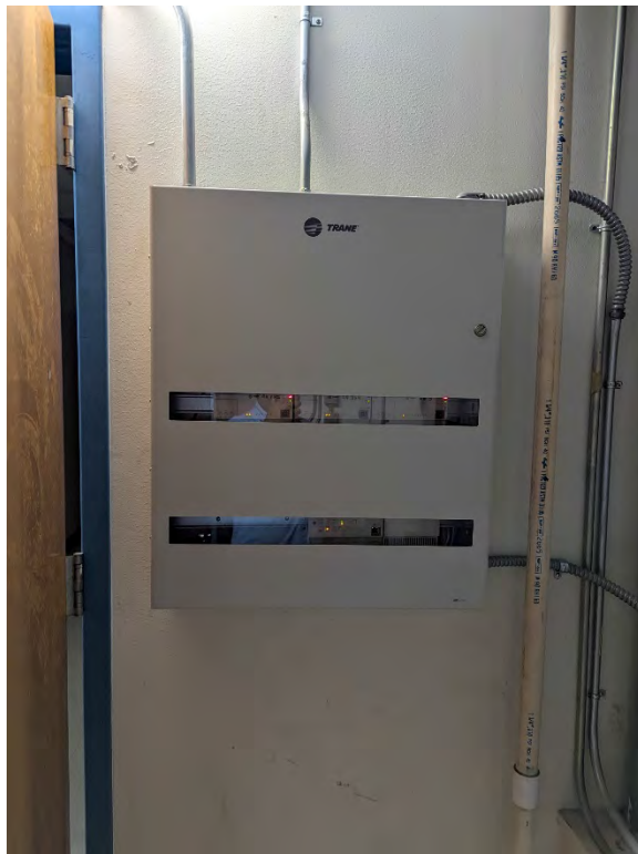
Figure 6. First floor controls cabinet
