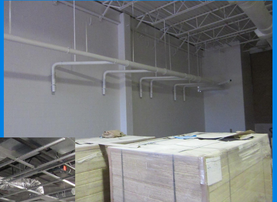
Dust Collector ducts
