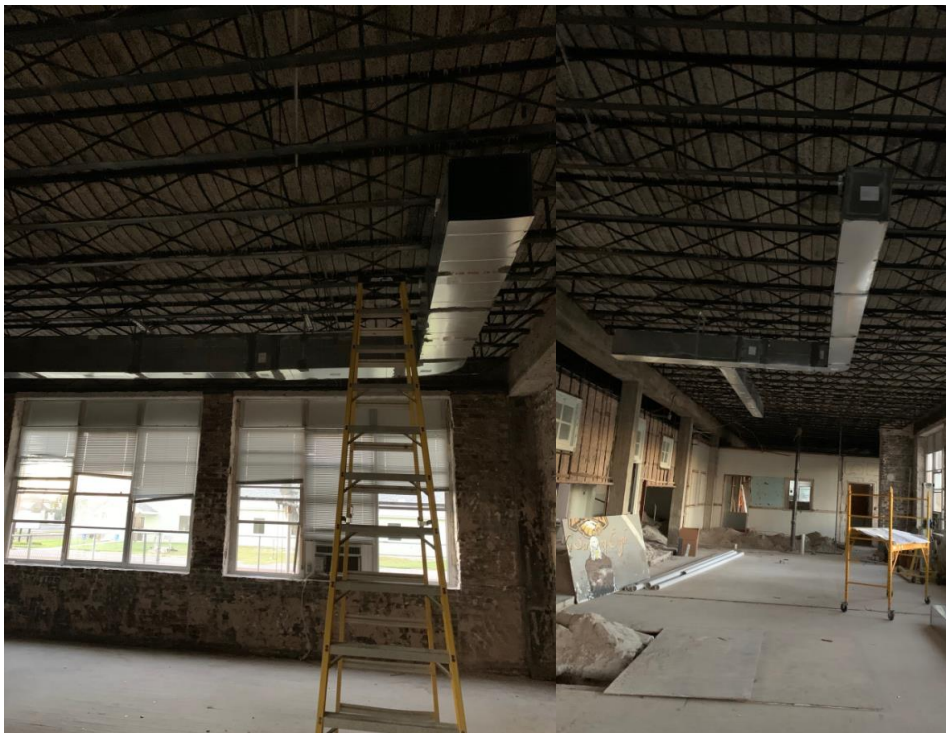
Above, new air ducting is being installed in what will be the administration offices.
