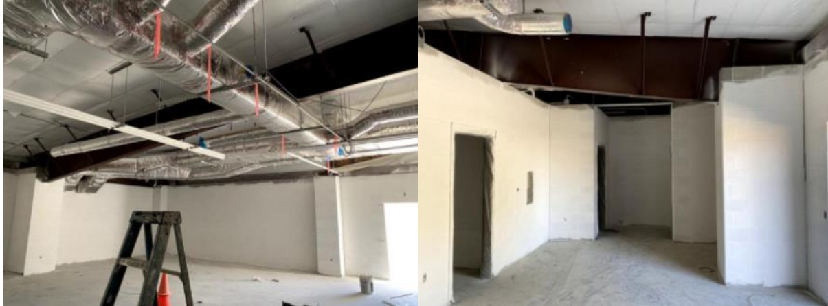
Above the new replacement Gold Gym is moving right along on schedule. The pictures above are from the dressing room areas.
