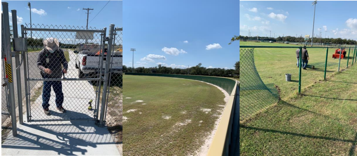
Top left John Crady adjusts to the closer for the pedestrian gate that leads out to the tennis courts. Top middle, the outfield for the softball field is completed. Top right, the work to replace the baseball outfield fence has begun.
