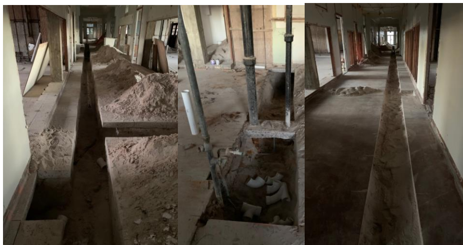
Above you can see where NorthStar contractors had to saw cut the slab to install new plumbing in what will eventually be the new administration offices.
