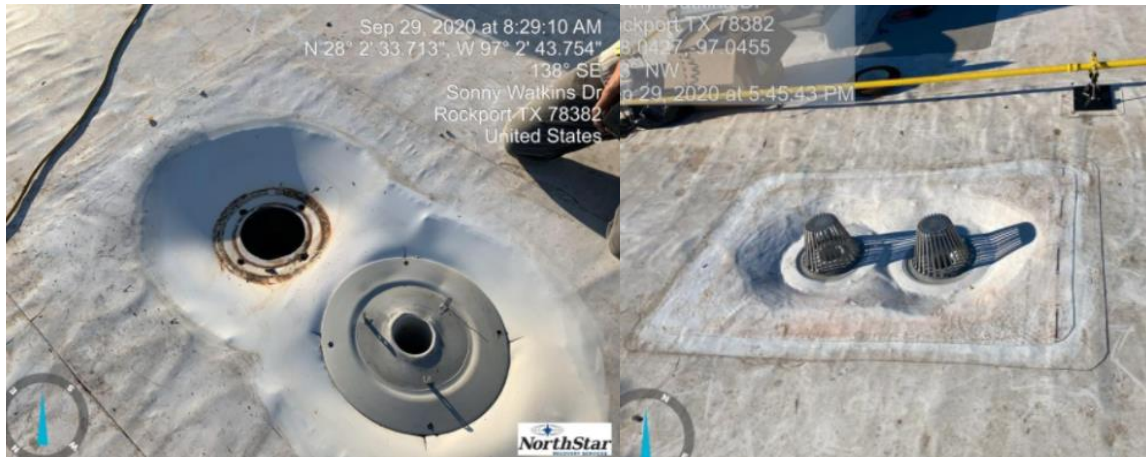
Above, FSR roofing completed several roof drains at RFHS so that the trash cans and water divertors could be removed.
