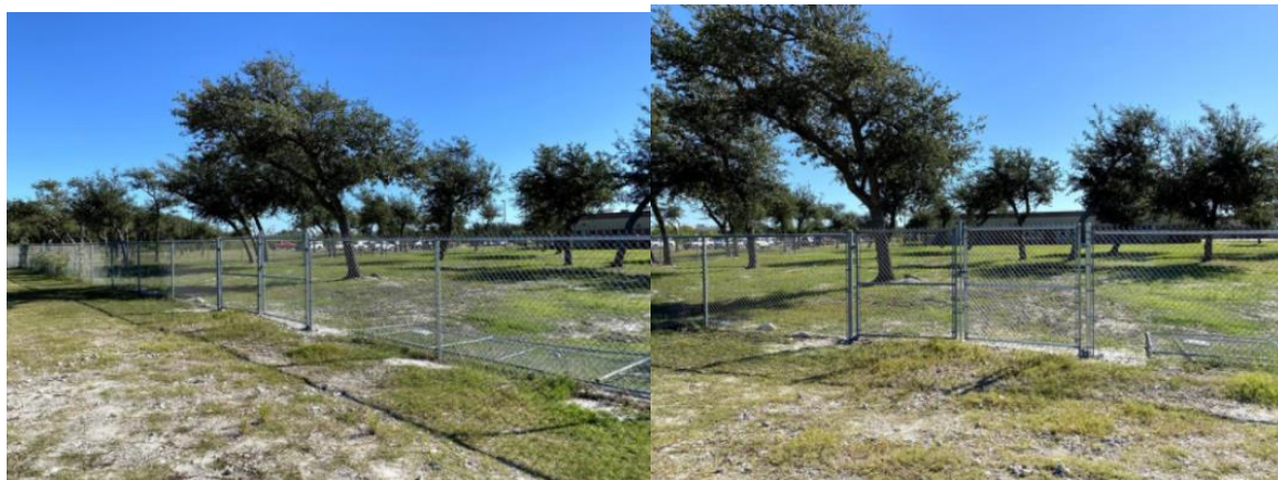
Above, new chain link fencing and new gate installed between RFMS and the Soccer practice field. This was done by contractors working for NorthStar and was damaged by Hurricane Harvey.
