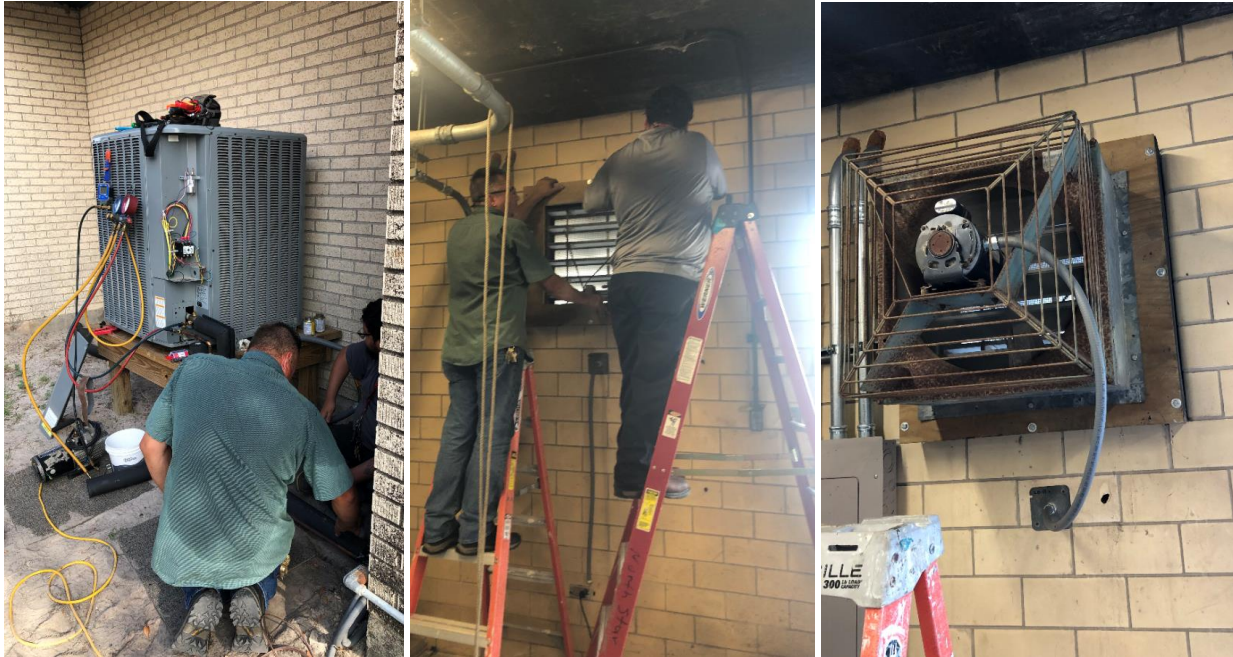
Above left, Larry Schindler and Dymond Garcia relocate an AC condensor unit at the Green Gym and above center and right, Larry and Dymond install a replacement vent fan for the Little Live Oak Chiller Room.
