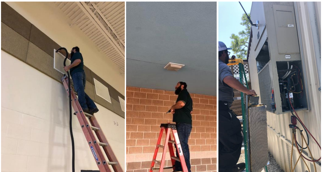
Above left, Carlos Leal vacuuming the air intakes inside the LOLC Gym. Above center, Carlos Leal replacing light bulbs on LOLC Front Porch. Above right, Dymond Garcia services an AC unit on one of the FLC portable classrooms. Carlos and Dymond are not afraid to climb a ladder!
