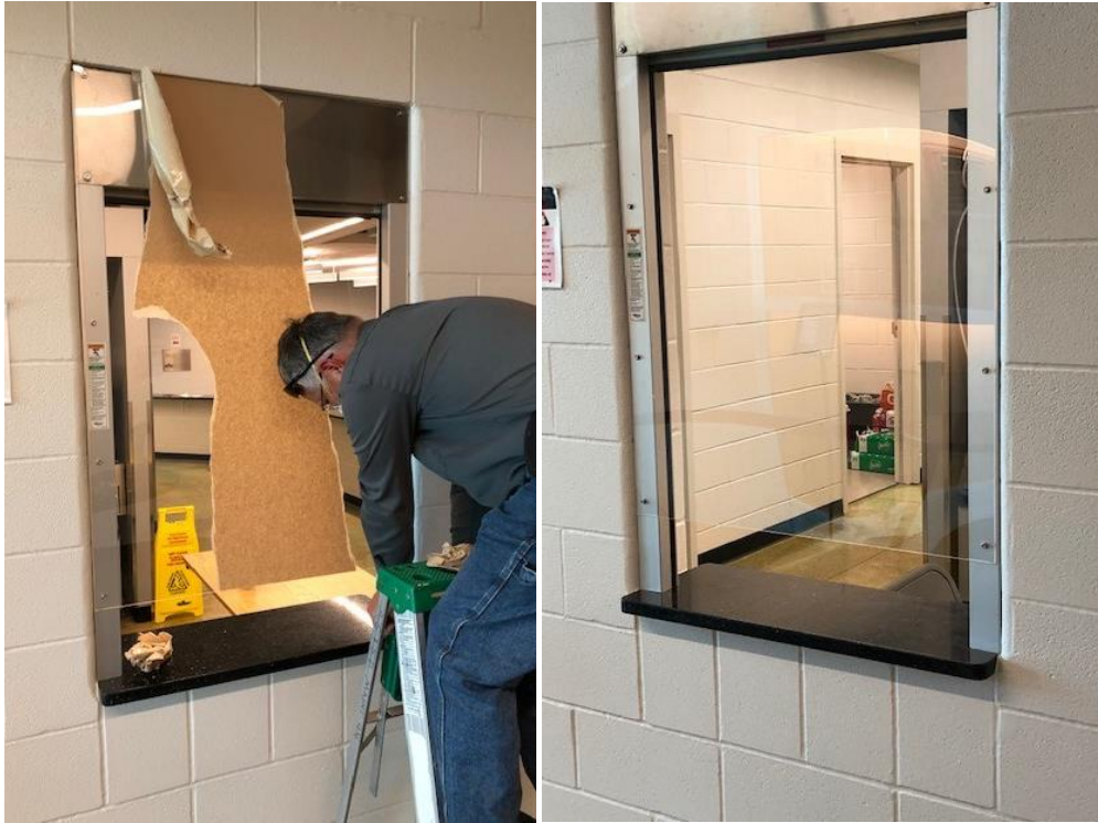
Above you can see where ACISD Maintenance Tech Kyle Bradley and John Crady installed plexiglass over the ticket window in the competition gym.
