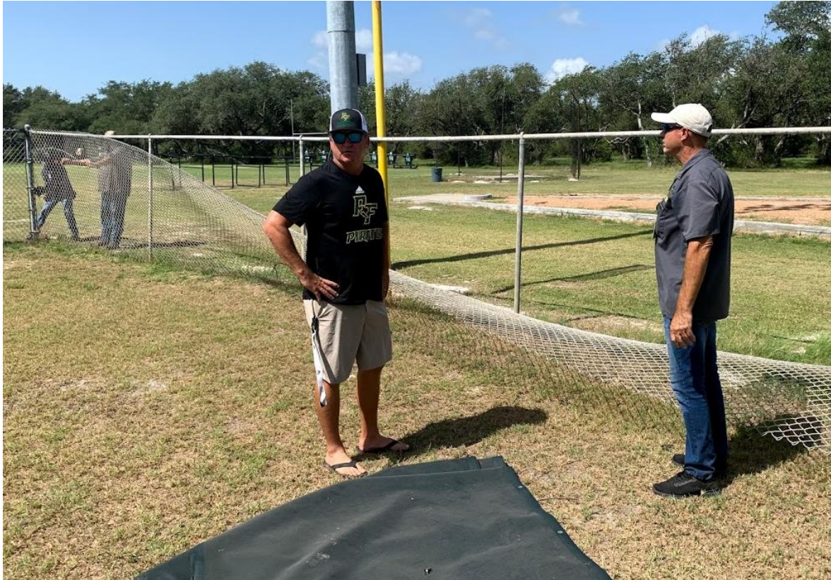
Athletic Director Jay Seibert oversees the removal of chain link fencing and the plan to assemble the new fence for the softball field.
