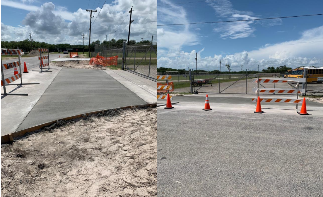
Above you can see the newly poured entrance to transportation that had to be cut in order to install underground drainage.
