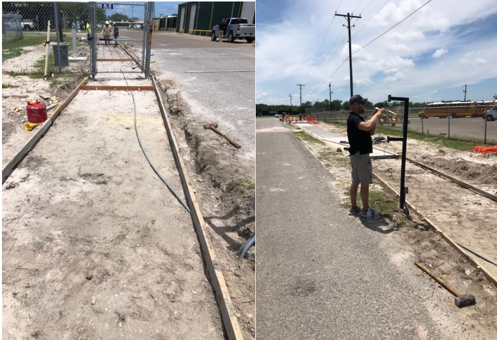
Above left, the sidewalk framing was in the works for the pedestrian sidewalk near the HS gate. Above right, Mike Nowotny works on the rerouting of the card readers after the rerouting of the cables was needed.
