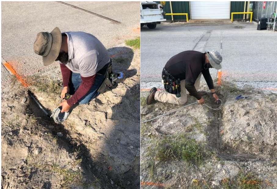
Top left Carlos Leal rerouting cables for the HS gate which had to be moved for the sidewalk pour. Top right, Dwayne Solis also working on the HS gate cable rerouting project.
