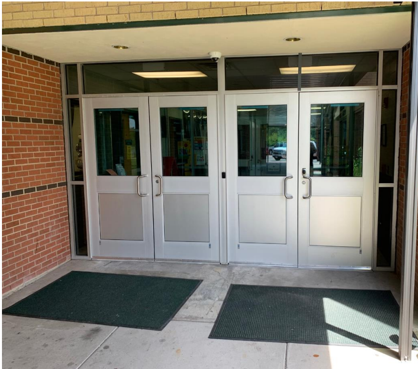
Completed front doors to RFMS paid for with a TEA Grant for safety and security.
