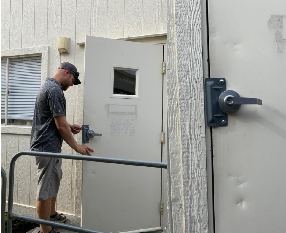
Above left, Mike Nowotny installs door latch guards on both doors to the construction trailer that will be housing Dina Hill and Joey Patek. The doors were very easy to open with a screw driver or pocket knife without the guards. They are now secure.
