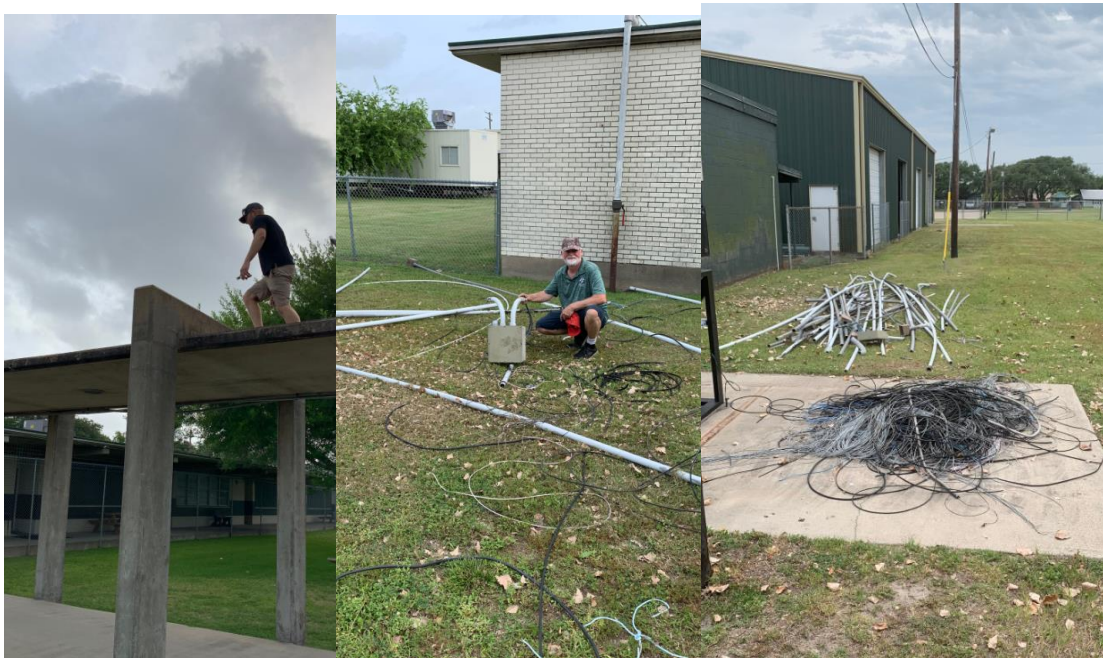
Above left, Mike Nowotny on the roof at old Rockport Elementary campus that is currently housing admin. The job was to remove as much pipe and cabling from up there that is no longer needed so that to make the job easier for the roofers which are soon to be on site. Above middle, John Staples, who likes to deer hunt, posing with a nice PVC pull box with some nice schedule 40 antlers.
