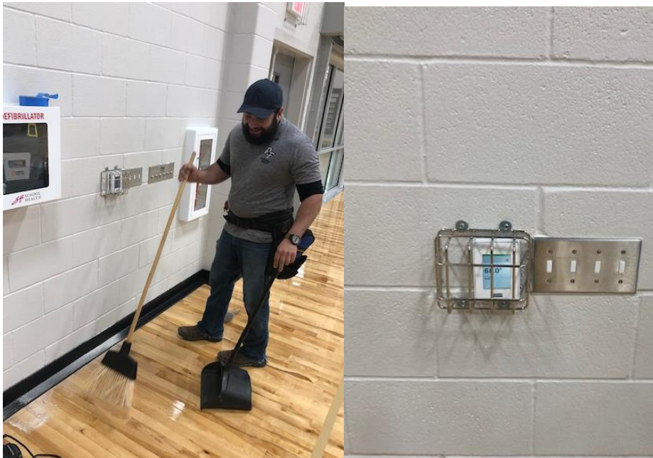
Above, Carlos Leal is happy to cleanup after installing a protective cage around this thermostat in the new gym.
