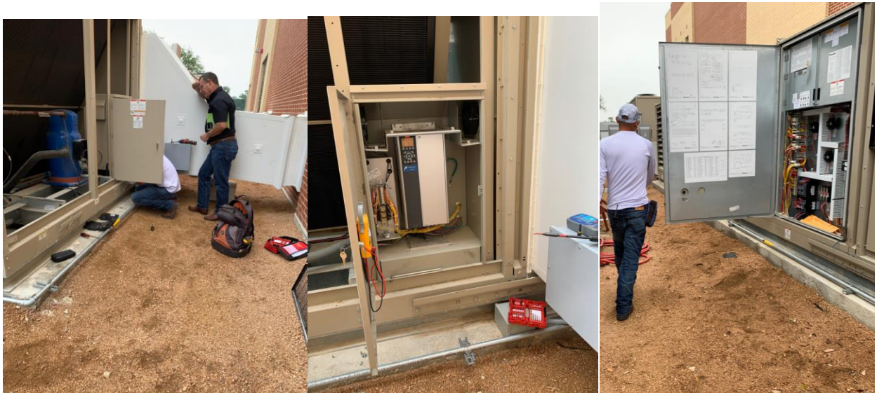
One of the 50 Ton package units for the new competition gym was failing and making a loud noise. The problem ended up being a faulty compressor drive which was covered under warranty.
