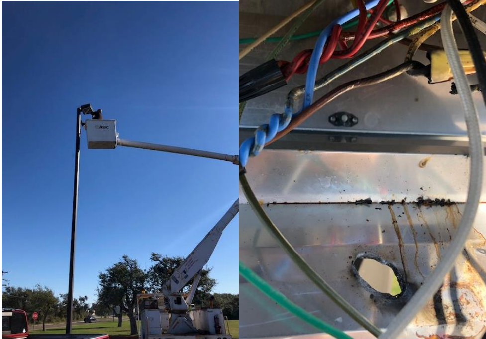
Above left, Dwayne Solis uses the districts bucket truck to repair a light in the front MS parking lot. When he got up there, he found where wires were burnt up causing an open to occur so the light wouldn't work. Repairs were made and all is good.
