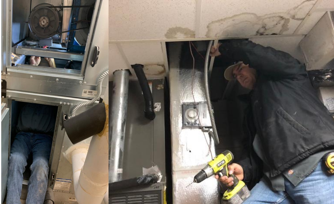
Top left, Lead AC Technician – Tom Hill squeezes into a tight space inside of the Air Handler Unit for LOLC Offices. Tom has been an awesome addition to our team. He has many years of experience and is not scared to do whatever it takes to get the job done. Top right, Maintenance Technician – Robert Miller repairs some ceiling grid in one of our mechanical rooms.
