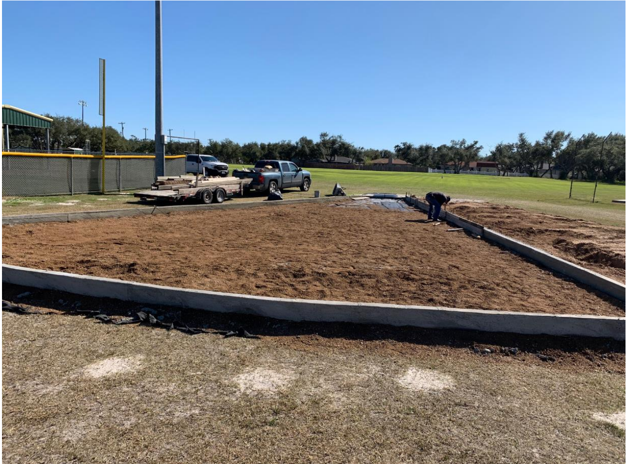
Construction is near completion of new shotput pit. Above you can see the contractor removing the forms from the newly poured concrete wall.
