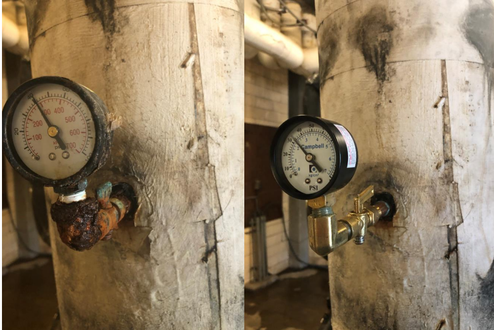
Above you can see a before and after photo of the pressure gauge that was replaced on the chiller out at Little Live Oak.
