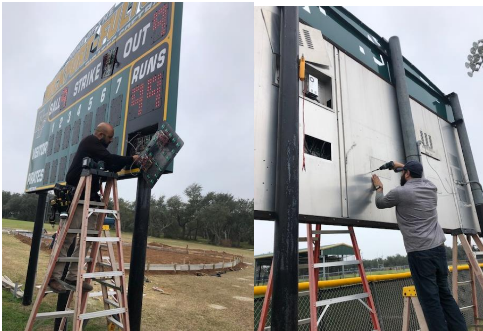
During our weekly preventative maintenance check of the scoreboards, we found that our outs and runs digits were not working. It was definitely a process to troubleshoot exactly what the issue was. The problem was a bad distribution plug in one of the false digits behind home digit panel. We replaced it with one we keep on hand.
