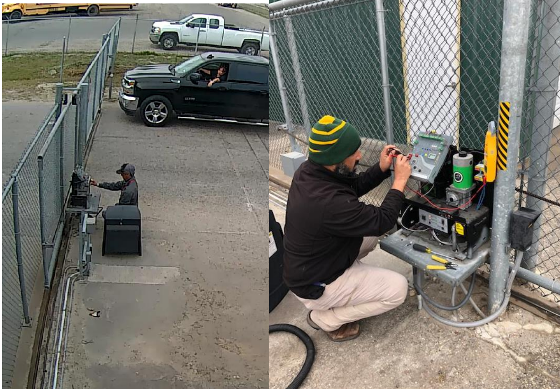
Gate wouldn't open or close. After taking a few readings we determined that the fuse was good but the fuse holder had some black corrosion built up over the yard in the cylinder case. Cleaned it out and it started working. Above left, you can see Andy Dominguez trying to get the gate to open. Above right, Dwayne Solis diagnosing the problem and repairing the motor.
