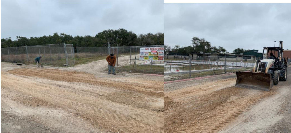
Andy Dominguez, James Arambula are cleaning the curbs of road base that are being spread by tractor driver David Serna. This is to help a little with the potholes in that area.
