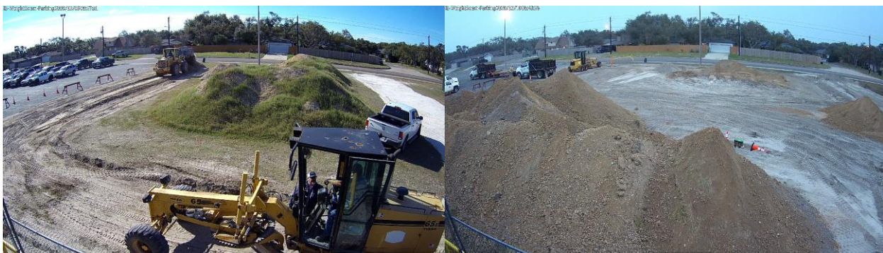
The mountain of base that we had stacked in the parking lot was slowly spread in that area. The base came from the parking lot where the new competition gym was built. I had TEAL construction pile it there instead of hauling it away. It really came in handy for this project and saved us quite a bit of money as well.
