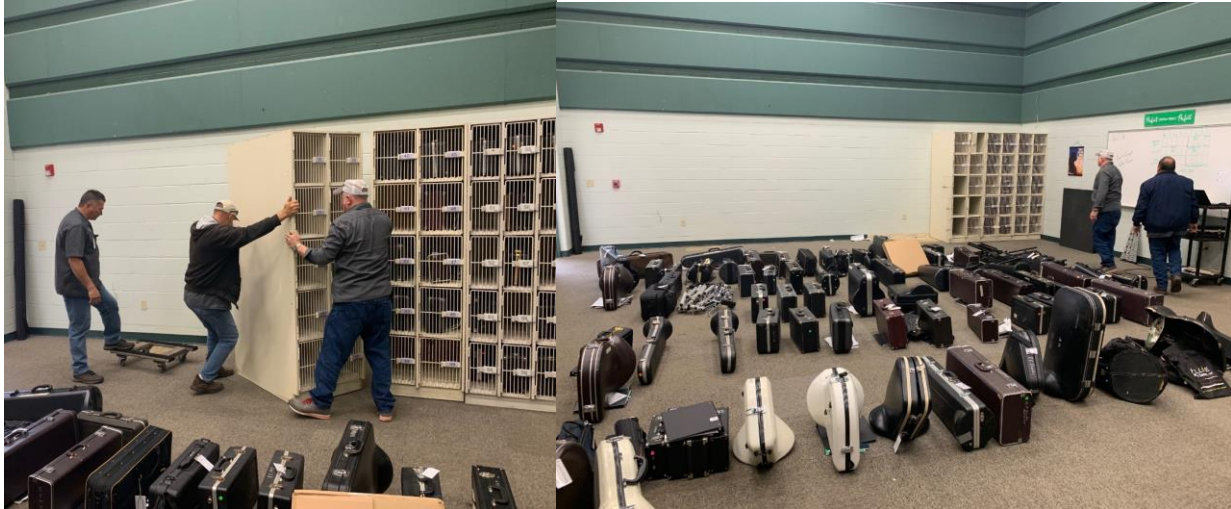
John Crady, Robert Miller, Larry Shindler and Floyd Mora remove the old band lockers that were damaged from hurricane Harvey from the RFMS band hall.
