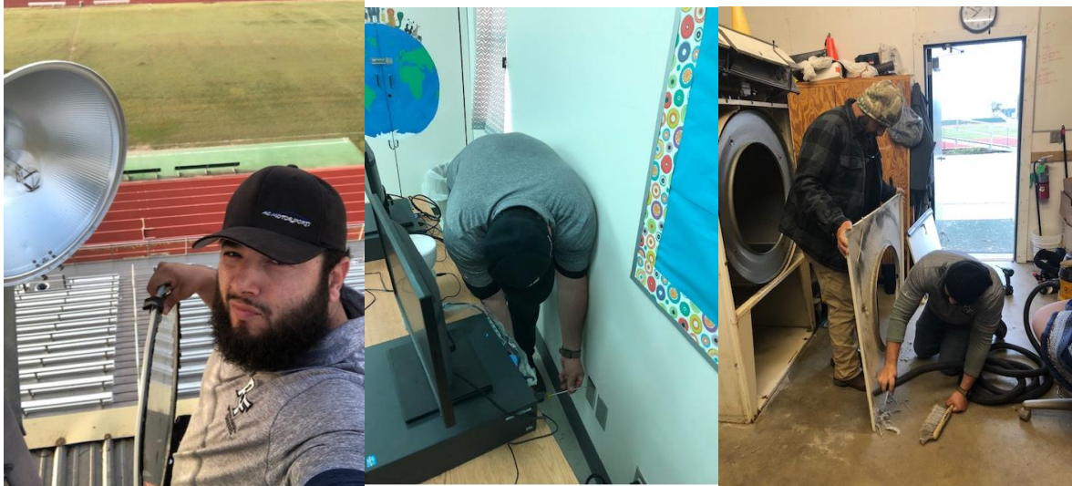
Top left, Carlos Leal replaces a bulb in the light setup on the press box so that our community can walk the track in the evenings. Top middle, Carlos Leal installed some blank faceplates over empty wall boxes and top right, Dwayne Solis and Carlos Leal dismantled the commercial dryer in the RFHS field house to remove a ton of lint so that we don't start any fires.
