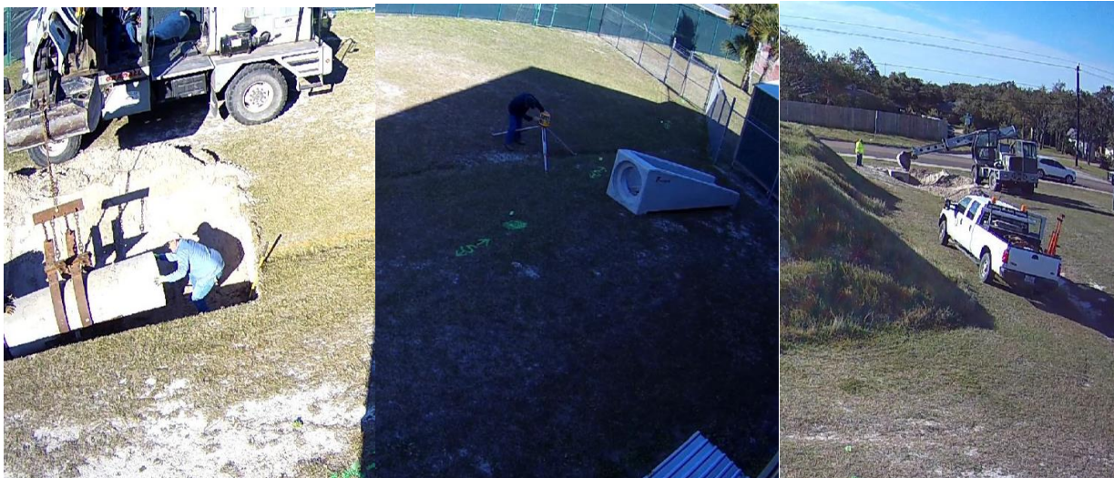
Above, the county began the work on expanding the RFHS parking lot. A drainage pipe was installed first.
