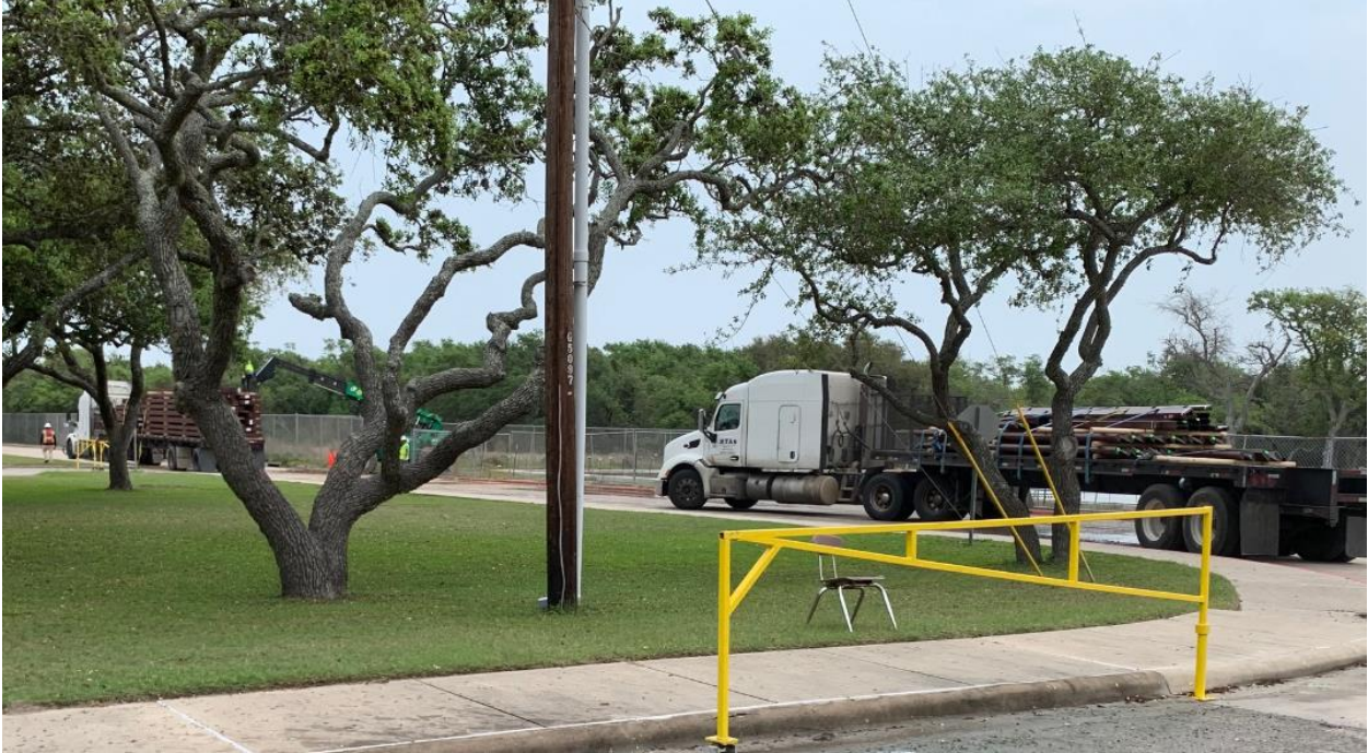
Steel arrived at the Gold Gym site on Tuesday, 4-7-2020 so things are looking up!
