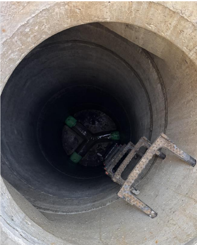
Photo 2: MH #3 debris in base
