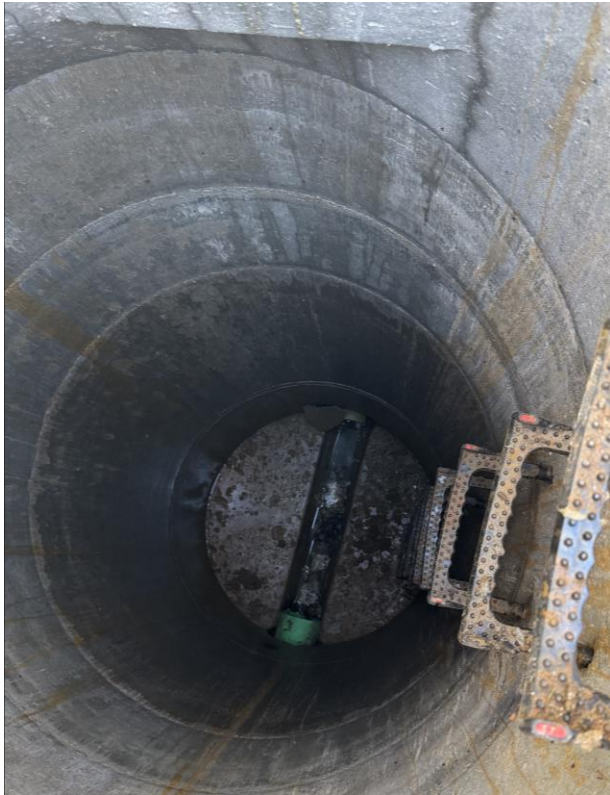
Photo 3: MH #4 debris in base
