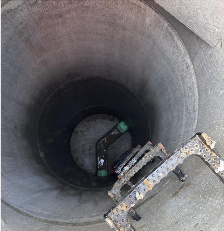
Photo 6: MH #9 debris in base
