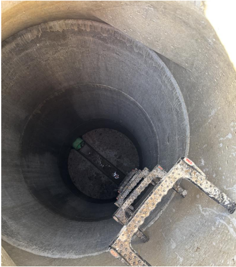
Photo 7: MH #10 debris in base
