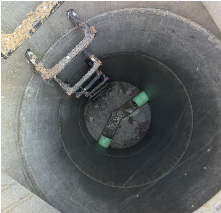
Photo 4: MH #7 debris in base
