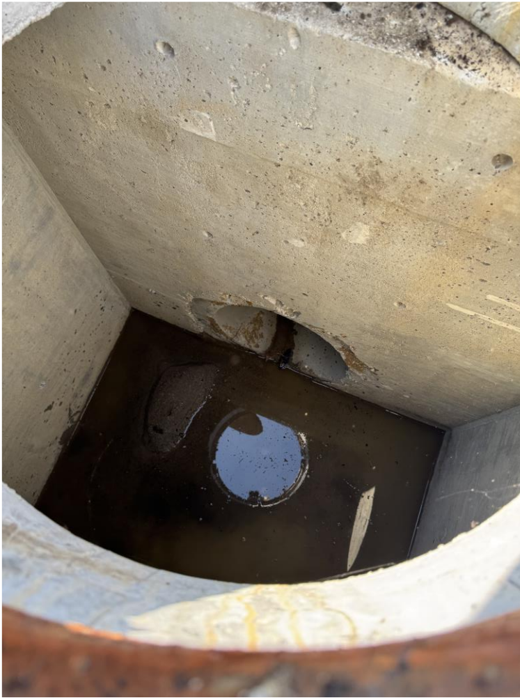
Photo 11: debris and standing water inside storm inlet 3 – floor of inlet is lower than pipe flowline creating standing water in inlet.
