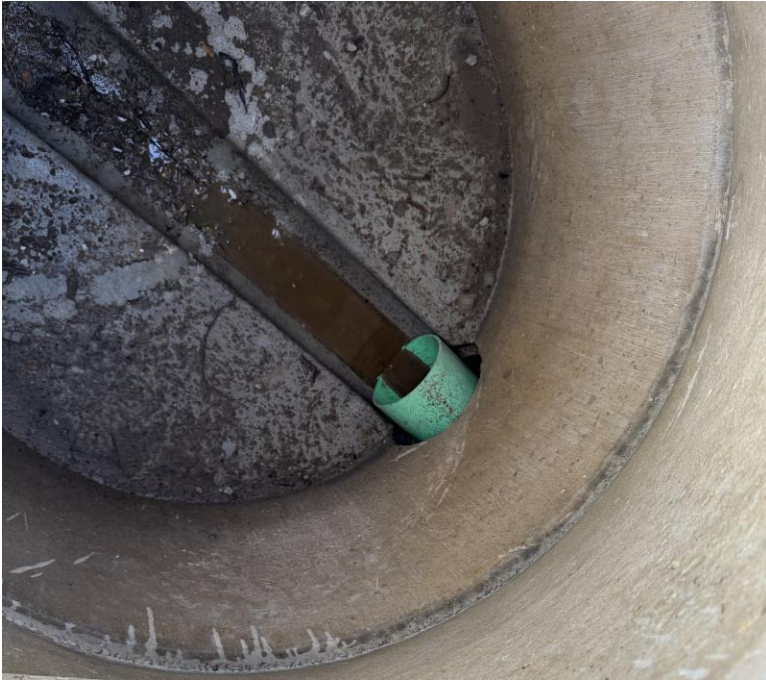
Photo 9: MH #13 debris in base & no grout inside MH around pipe
