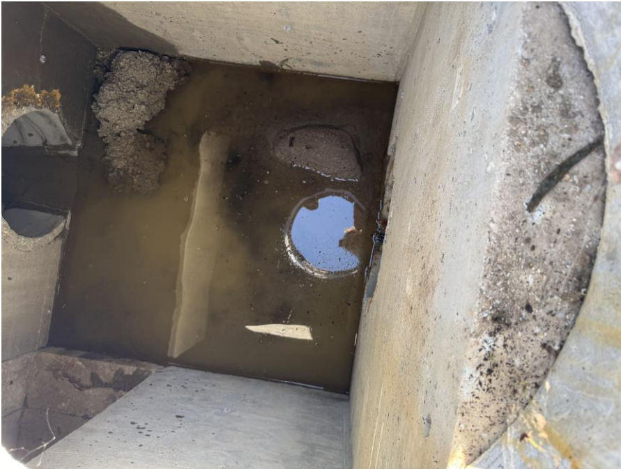
Photo 10: debris and standing water inside storm inlet 4
