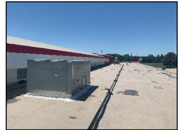
2 North RTUs with Gas Lines
