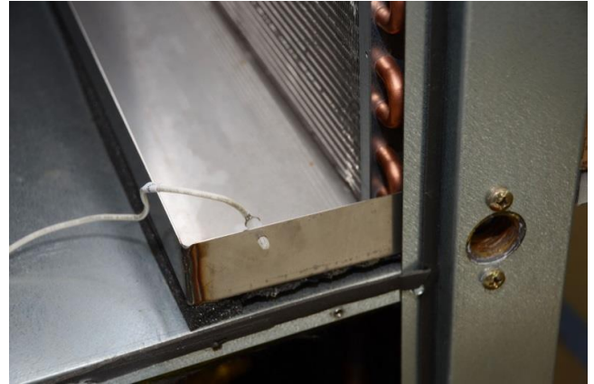
Condensate conductor connected to the condensate drain pan.
