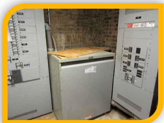
Main Distribution Panel
