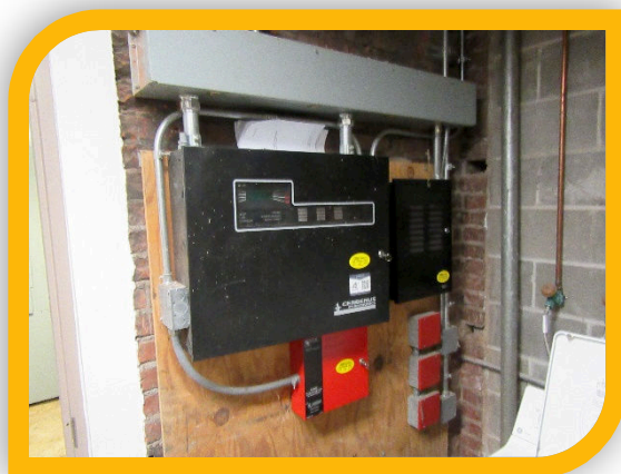
Fire Alarm System
