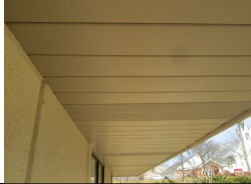
Soffit with code required lower vent area.
