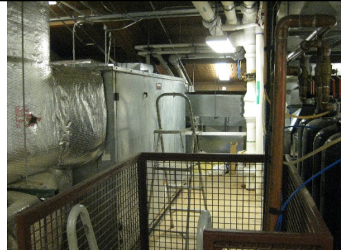
Existing energy recovery ventilator in attic space.
