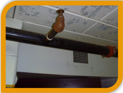
Fire Sprinkler System
