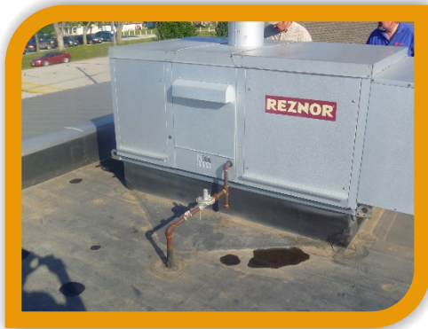
Make Up Air Unit
