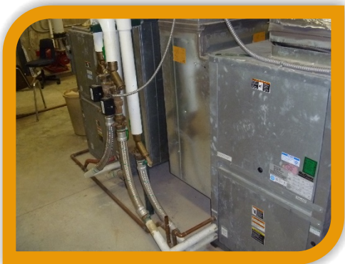
Water Source Heat Pump
