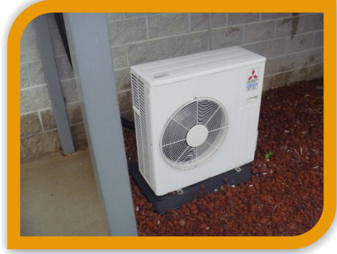
Ductless Split System
