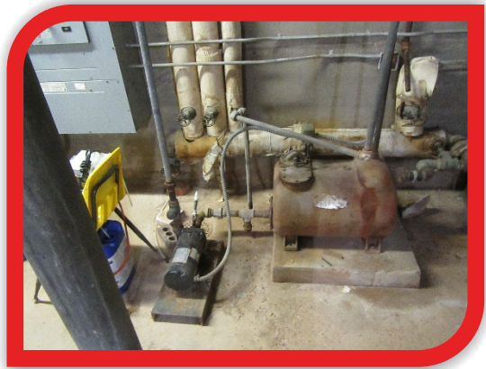
Steam Condensate Receiver
