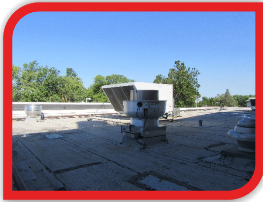
Roof Top Unit
