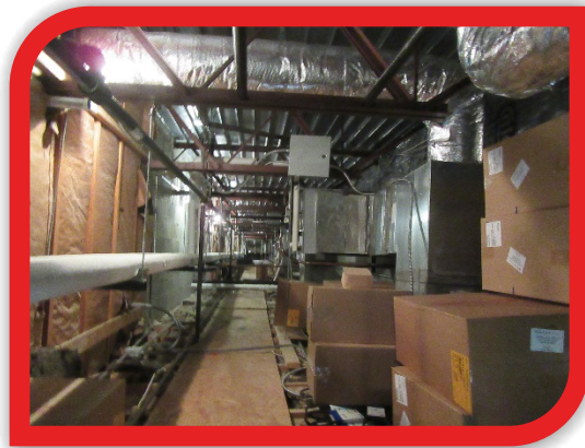
Elementary Mechanical Mezzanine
