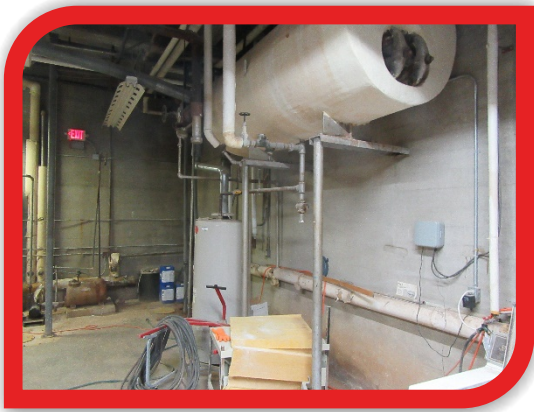
Hot Water Storage Tank
