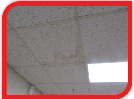
Elementary Water Stain
