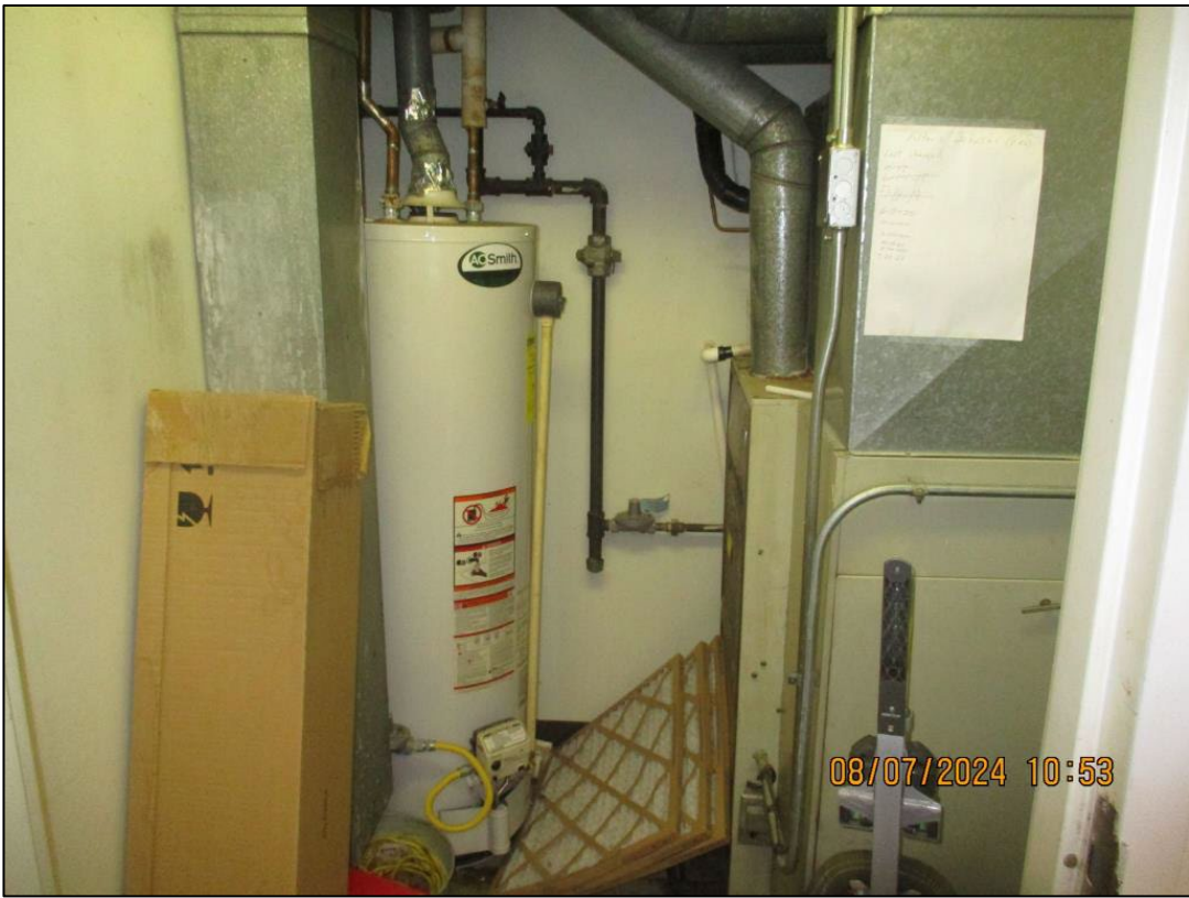
31009 Building- Furnace Room
