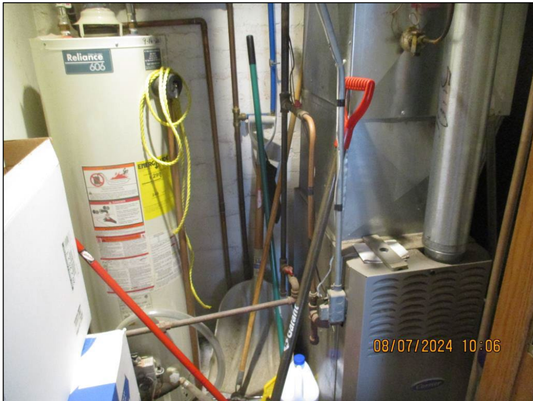
31001 Buiding- Furnance Room
