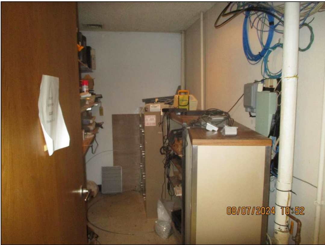
31009 Building- Mechanical Room
