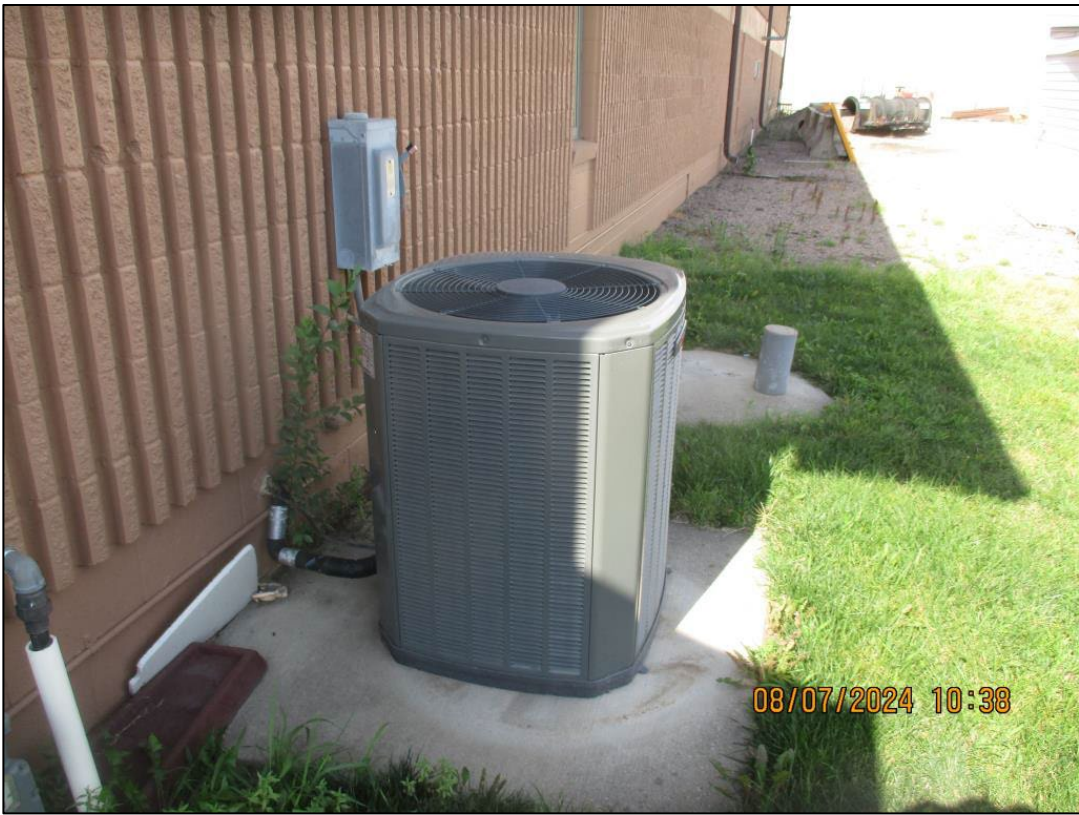
31009 Building- Central Air
