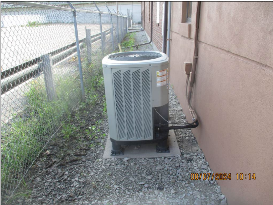
31001 Building- Central Air
