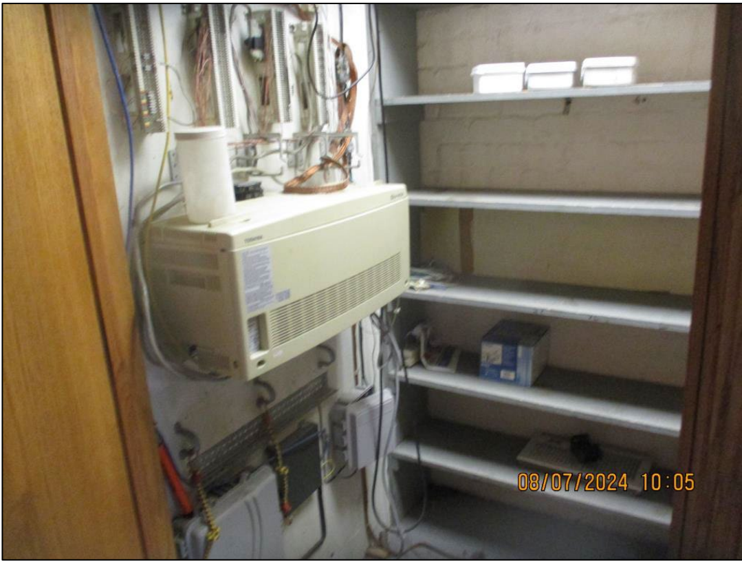
31001 Building- Electrical Room
