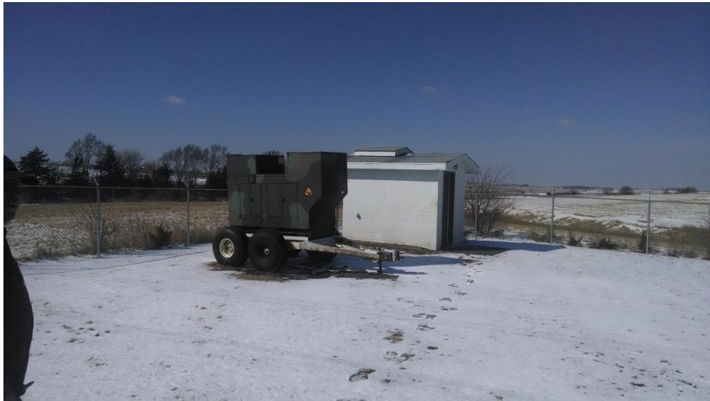
Figure 2-7: Well 76-1 (North Well)
