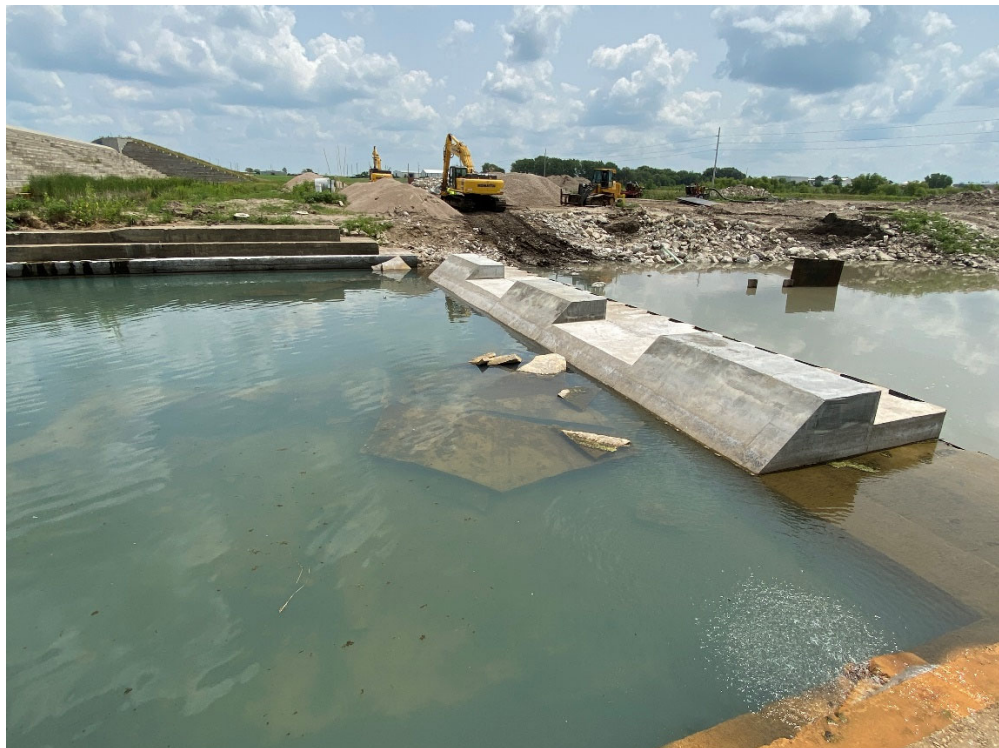
4 – Spillway apron surfacing after runoff event
