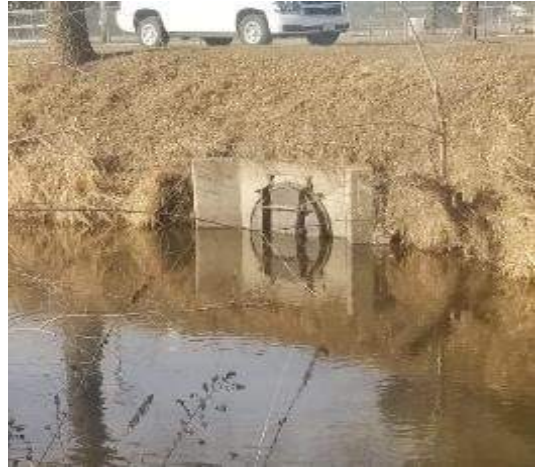
Picture 1: Flap Gate at Outfall 8
