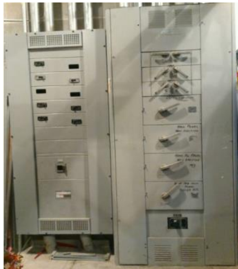
600A 3-phase services #2 and #3 ↑
