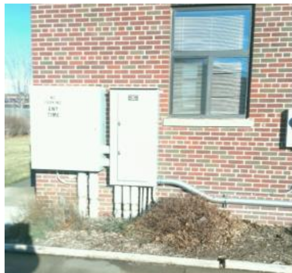
Campus electrical service ↑
