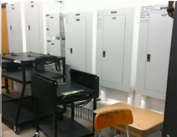
Panelboards for branch circuit distribution ↑
