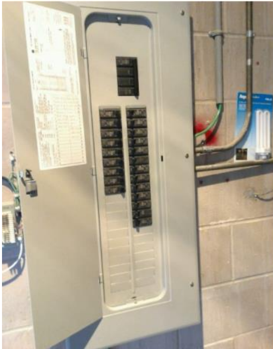
Service entrance loadcenter ↑
