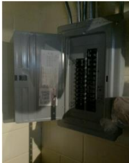
Basement sub panel ↑
