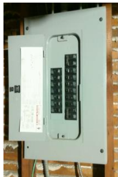
East basement sub panel ↑
