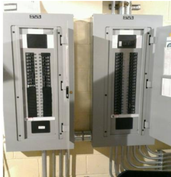
Rectory lighting panels ↑
