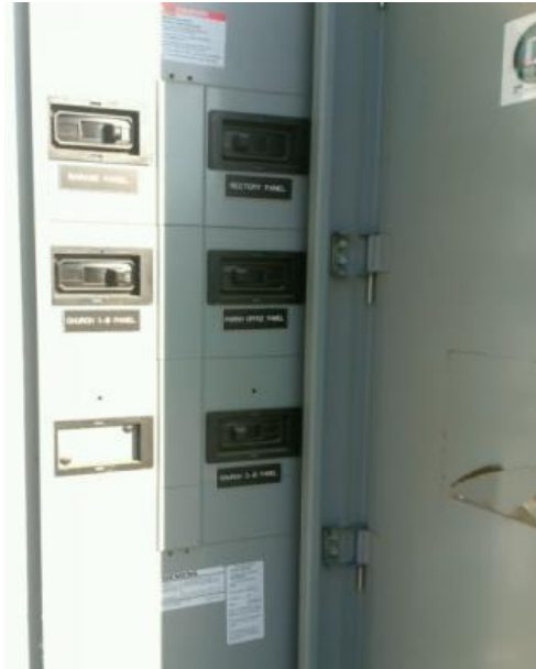
Campus distribution panel ↑
