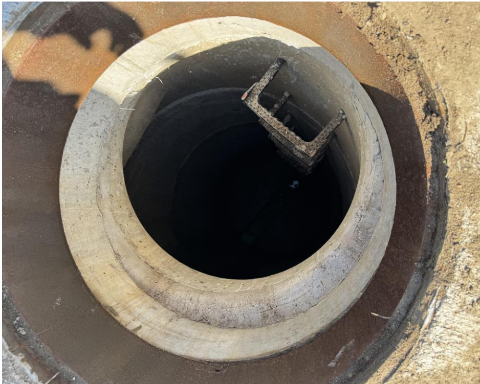
Photo 8: MH #10 adjustment rings not set on top of cone (about 2" off)
