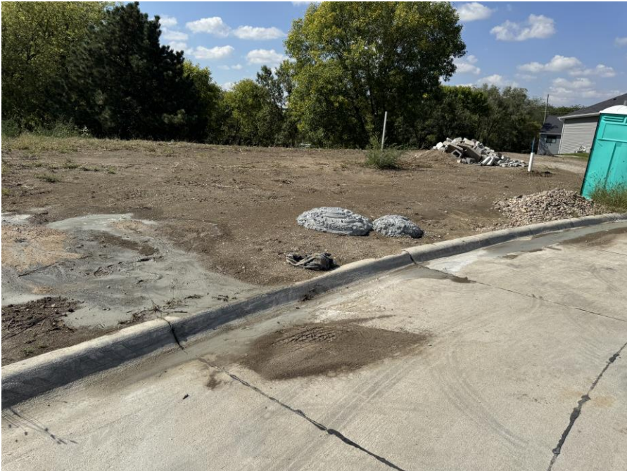
Photo 12: concrete washout on ground
