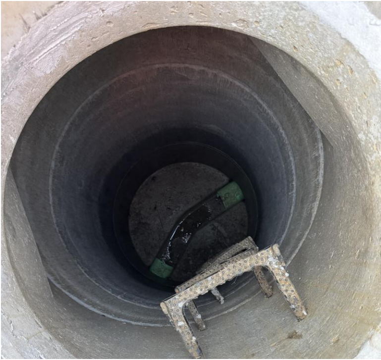
Photo 5: MH #8 debris in base
