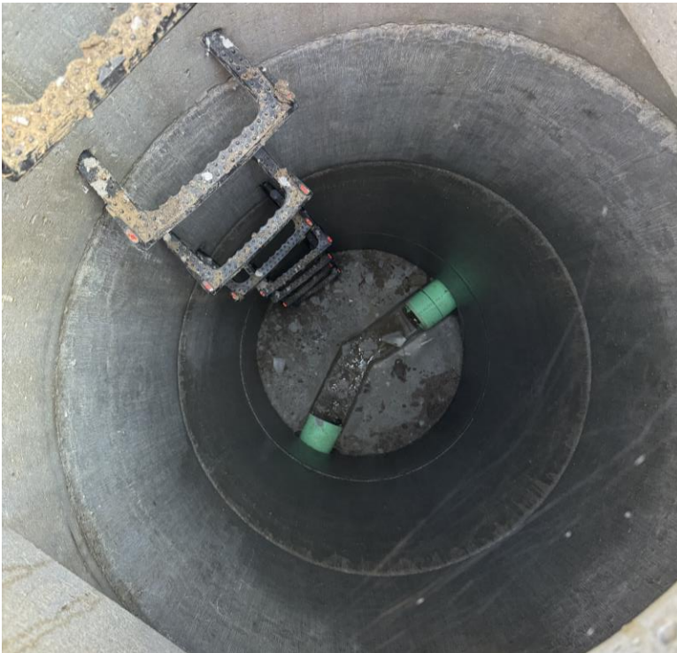
Photo 4: MH #7 debris in base
