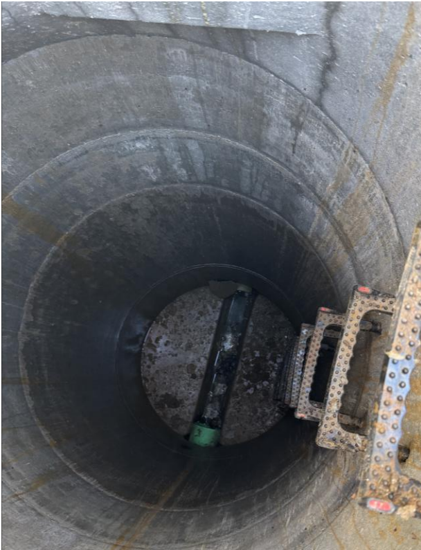
Photo 3: MH #4 debris in base
