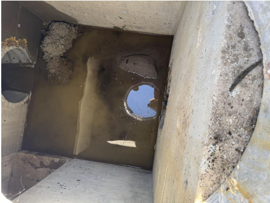
Photo 10: debris and standing water inside storm inlet 4
